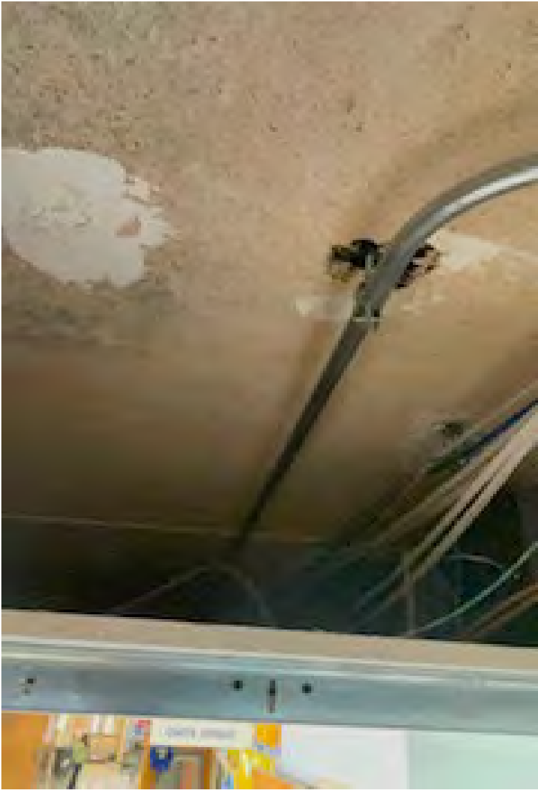
Asbestos Ceiling Texture
