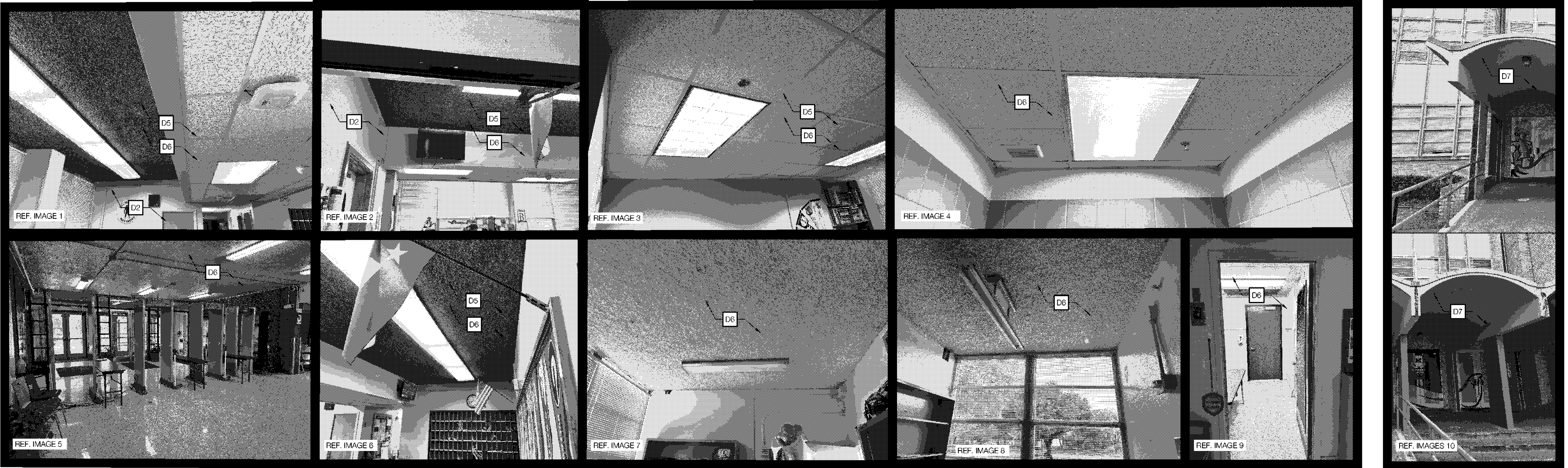
IMAGES ABOVE ARE INCLUDED FOR REFERENCE ONLY, IT IS THE GENERAL CONTRACTOR'S RESPONSIBILITY TO VERIFY ALL EXISTING CONDITIONS PRIOR TO CONSTRUCTION.
