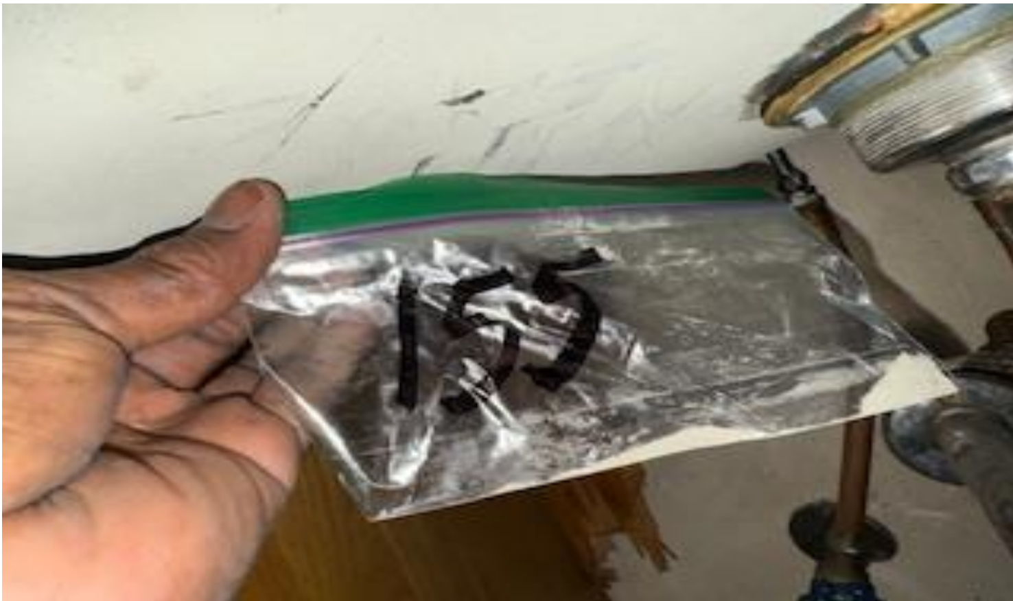
66 VIEW OF REPRESENTATIVE (TYPICAL) SAMPLE OF ACM WHITE SINK PUTTY LOCATED IN THE VESTIBULE ON THE 2 ND FLOOR IN A BUILDING AT THE THOMAS C. MARSH PREPARATORY ACADEMY
