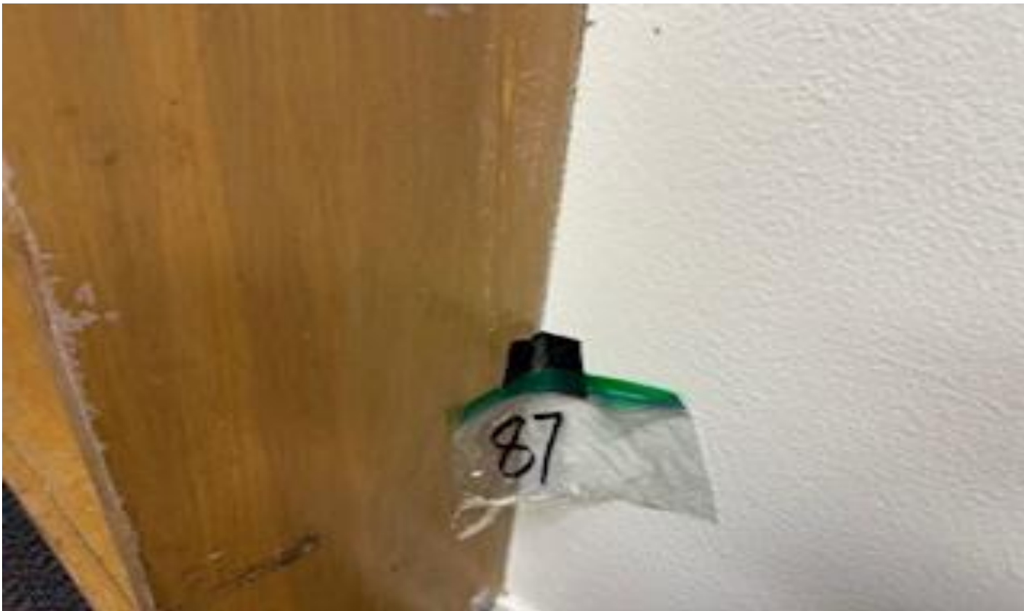
48 VIEW OF MORE REPRESENTATIVE (TYPICAL) SAMPLE OF ACM CAULKING ON CABINET WORKS LOCATED IN CLASS ROOMS AND ELSEWHERE THROUGHOUT THE BUILDINGS AT THOMAS C. MARSH PREPARATORY ACADEMY
