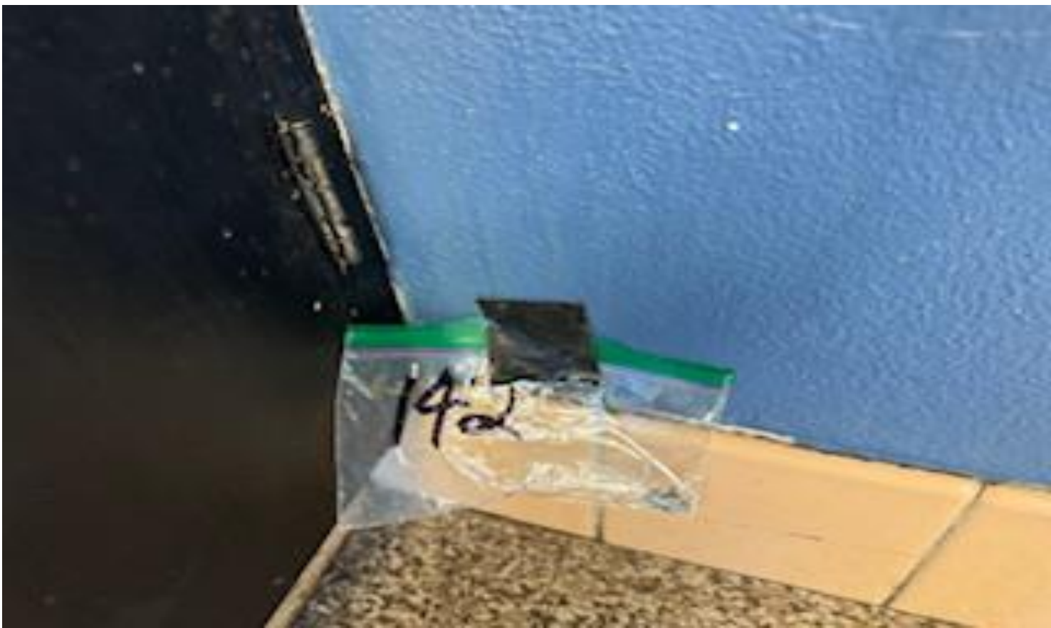
61. VIEW OF MORE REPRESENTATIVE (TYPICAL) SAMPLE OF ACM CABINET WORKS CAULKING LOCATED IN CLASS ROOMS AND OTHER FUNCTIONAL SPACES ON THE 2 ND FLOOR IN BUILDINGS AT THOMAS C. MARSH PREPARATORY ACADEMY
