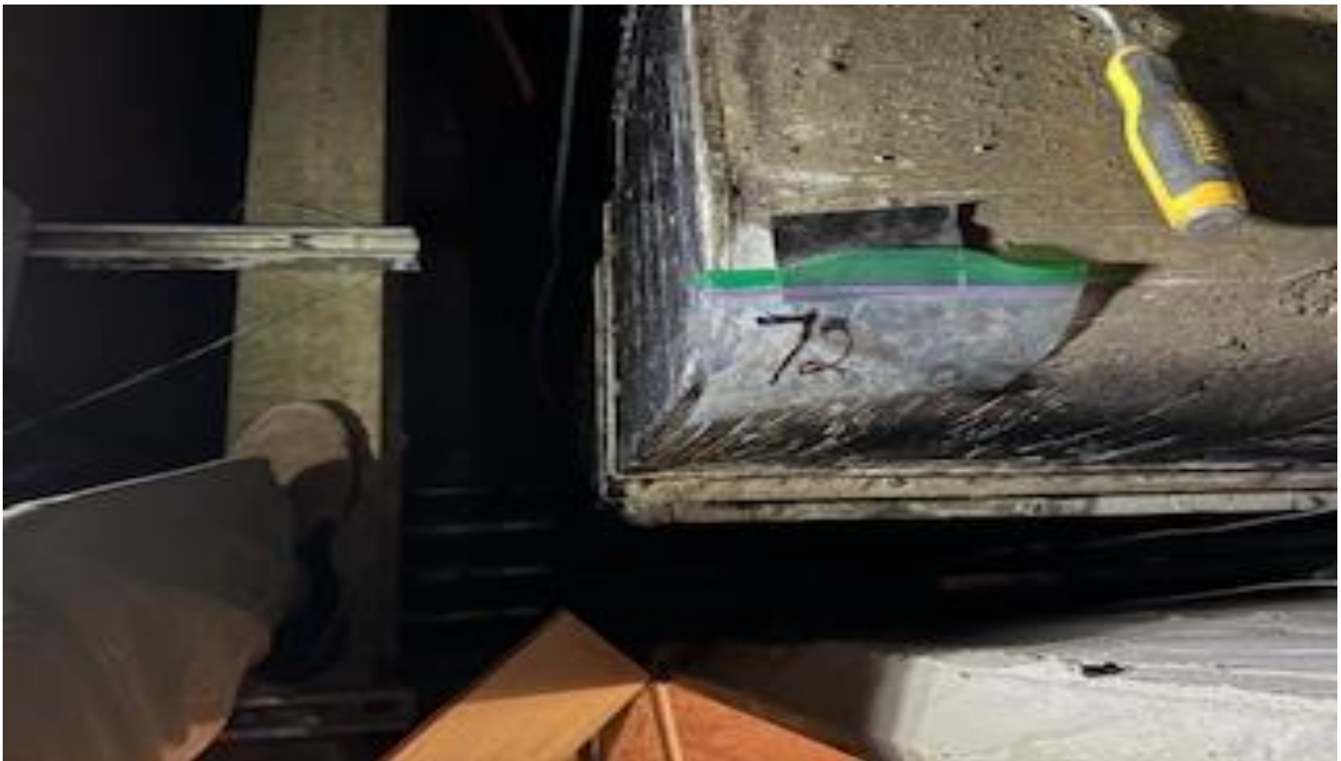
44. VIEW OF REPRESENTATIVE (TYPICAL) SAMPLE OF ACM THERMAL BLACK MASTIC ON METAL DUCT WORK LOCATED IN THE ELECTRICAL ROOM AND CRAWL SPACE UNDERNEATH BUILDINGS AT THOMAS C. MARSH PREPARATORY ACADEMY
