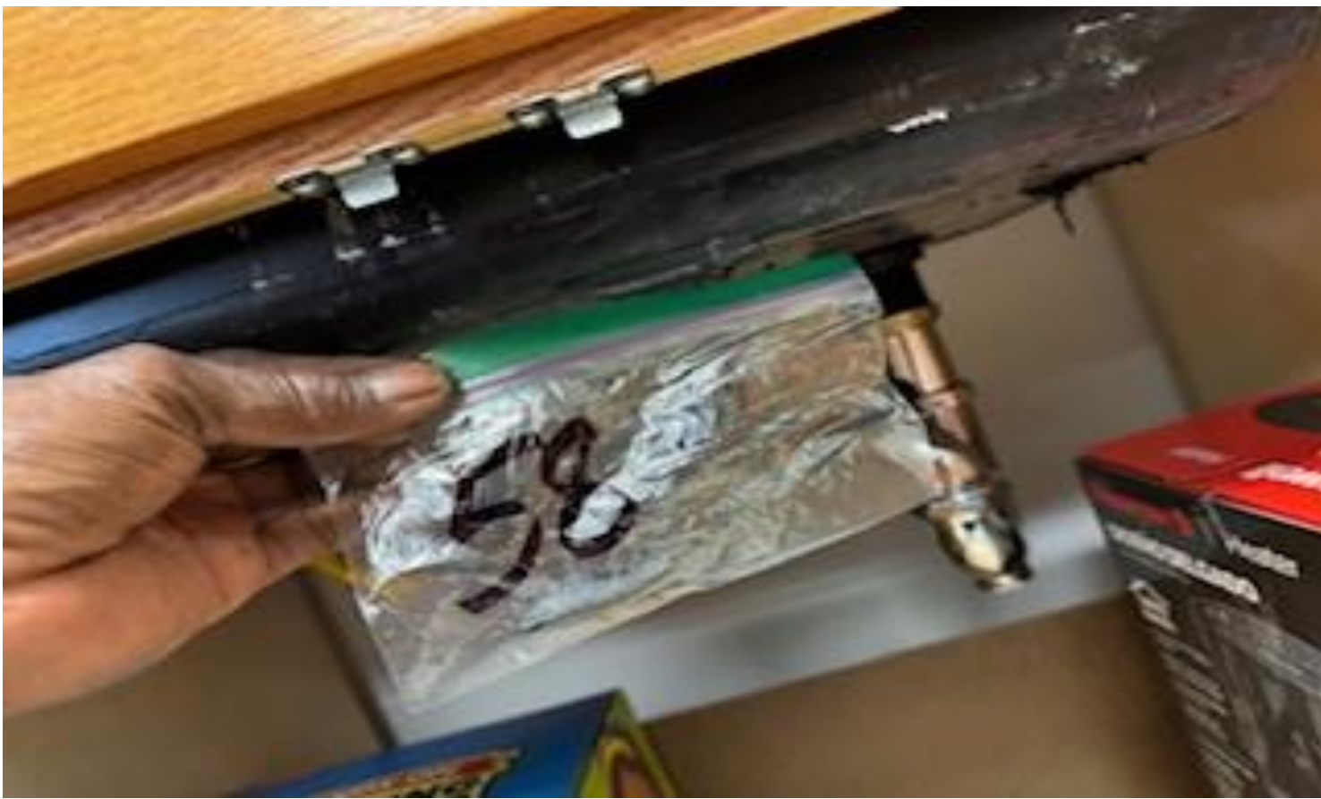
41. VIEW OF REPRESENTATIVE (TYPICAL) SAMPLE OF NON-ACM BLACK SINK PUTTY LOCATED UNDERNEATH VARIOUS HAND-WASH BASINS THROUGHOUT THE BUILDINGS AT THOMAS C. MARSH PREPARATORY ACADEMY
