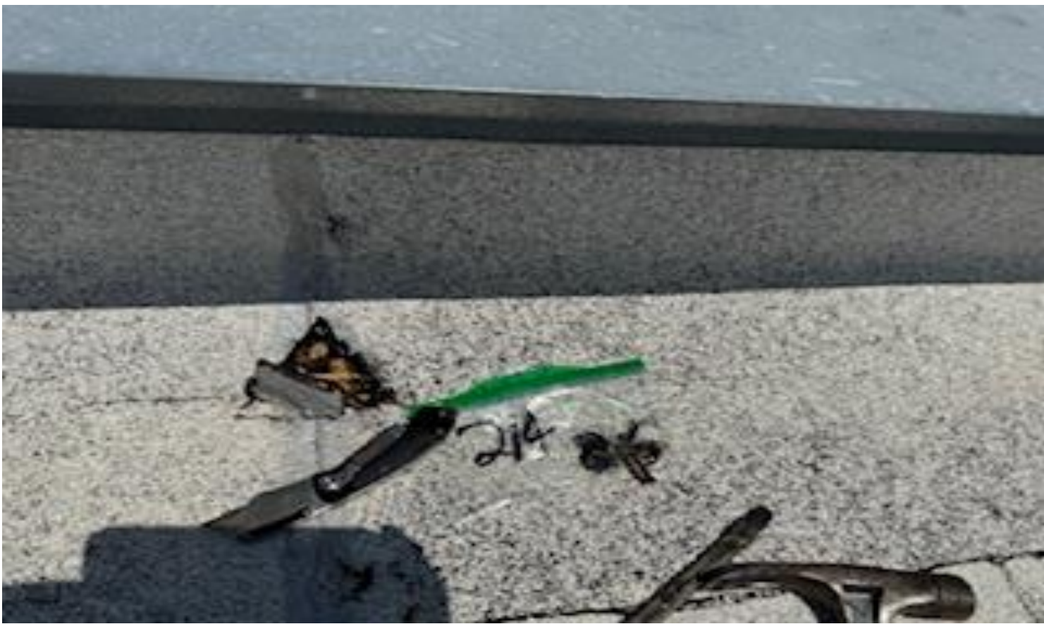
83. VIEW OF REPRESENTATIVE (TYPICAL) SAMPLE OF NON-ACM ROOF RIDGE BLACK MASTIC SEALANT LOCATED THROUGHOUT TOP ROOFS OF THE BUILDINGS AT THOMAS C. MARSH PREPARATORY ACADEMY
