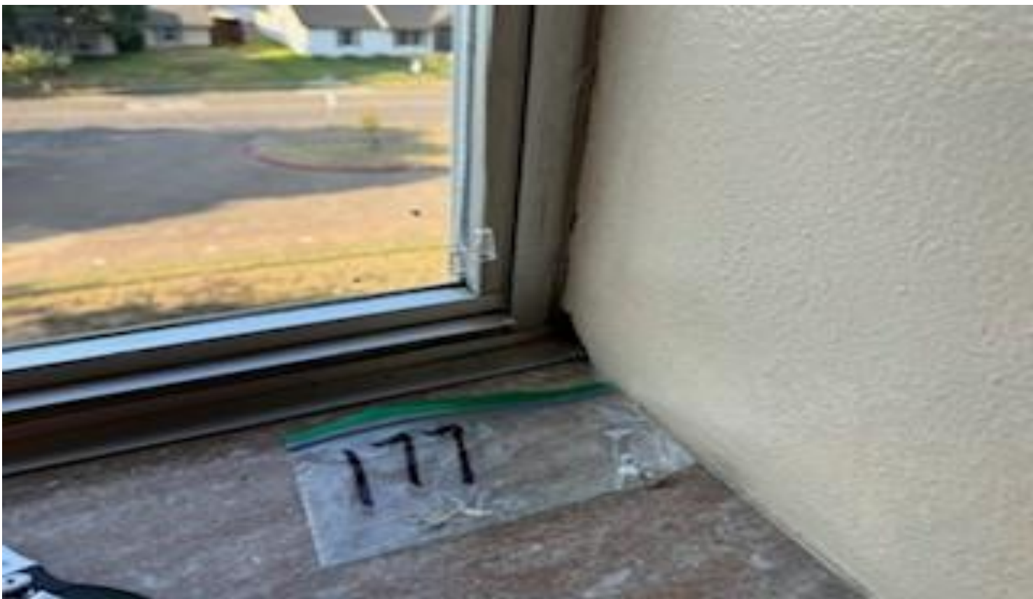
71 VIEW OF MORE REPRESENTATIVE (TYPICAL) SAMPLE OF ACM INTERIOR WINDOW CAULKING LOCATED THROUGHOUT THE INTERIOR 3 RD FLOOR WALL SURFACES IN BUILDINGS AT THOMAS C. MARSH PREPARATORY ACADEMY
