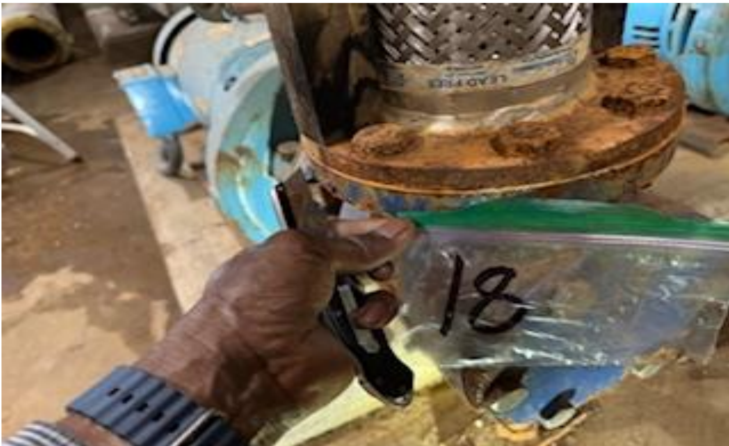
14. VIEW OF REPRESENTATIVE (TYPICAL) SAMPLE OF NON-ACM GASKET INSULATION LOCATED IN THE BASEMENT BOILER/SPRINKLER ROOM IN A BUILDING AT THOMAS C. MARSH PREPARATORY ACADEMY
