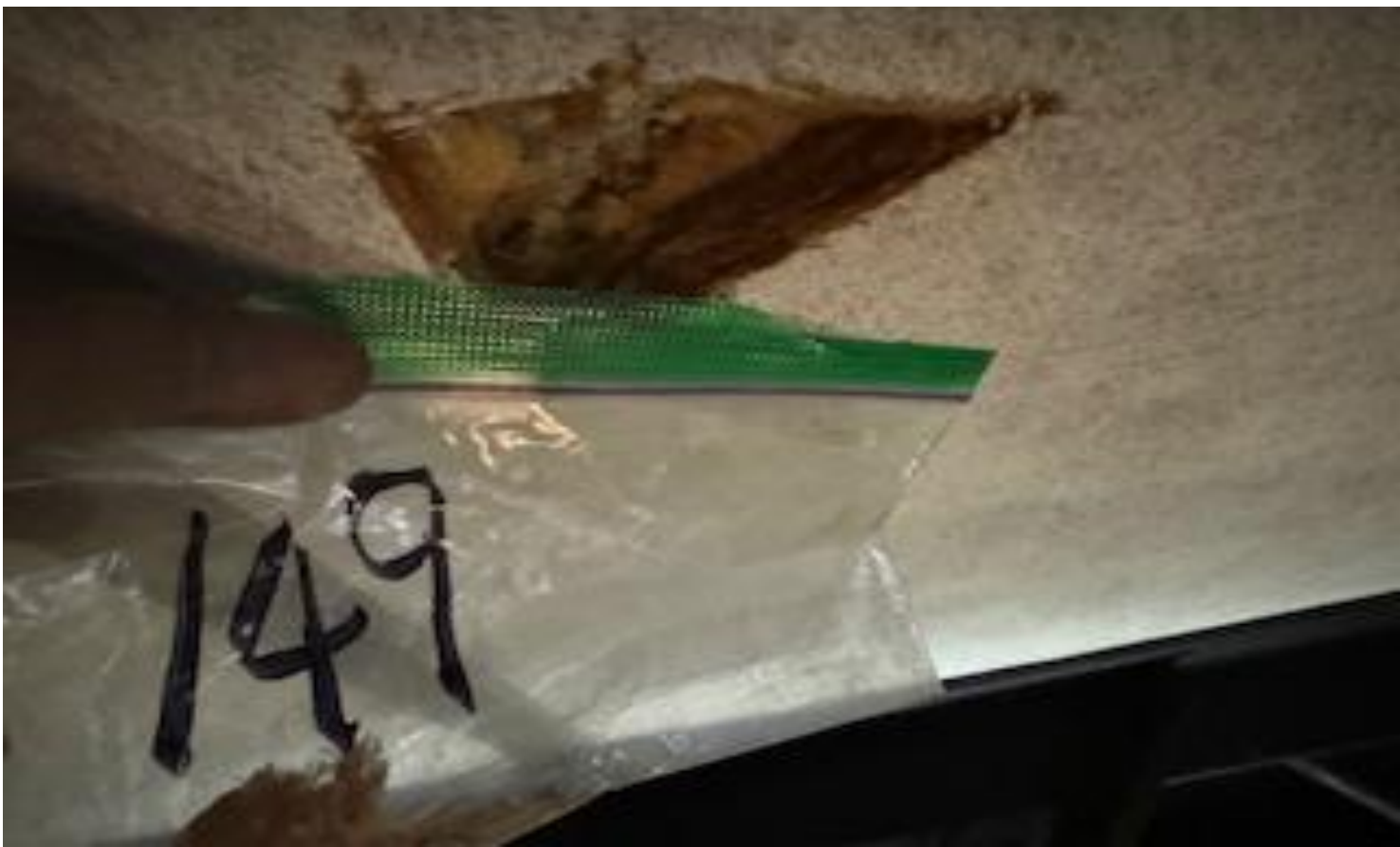
65 VIEW OF MORE REPRESENTATIVE (TYPICAL) SAMPLE OF ACM SPRAY-APPLIED CEILING (SAC) TEXTURE LOCATED ON INTERIOR 2 ND FLOOR CEILING SURFACES IN BUILDINGS AT THOMAS C. MARSH PREPARATORY ACADEMY
