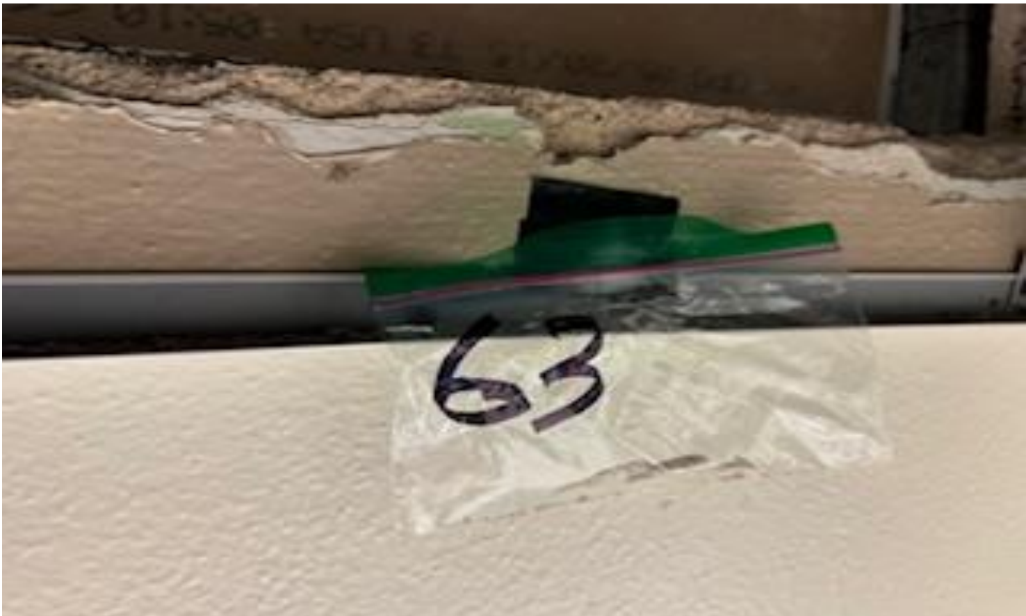
42. VIEW OF MORE REPRESENTATIVE (TYPICAL) SAMPLE OF NON-ACM PLASTER WALL LOCATED THROUGHOUT INTERIOR WALL SURFACES IN BUILDINGS AT THOMAS C. MARSH PREPARATORY ACADEMY
