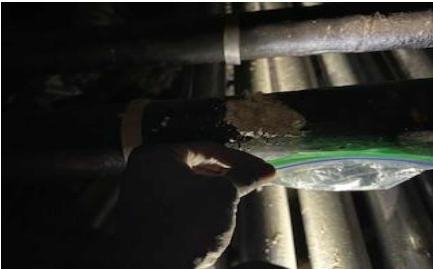
77. VIEW OF MORE REPRESENTATIVE (TYPICAL) SAMPLE OF ACM THERMAL SYSTEMS INSULATION (TSI) ON PIPE-RUNS LOCATED IN THE CRAWL SPACE UNDERNEATH ALL BUILDINGS AT THOMAS C. MARSH PREPARATORY ACADEMY
