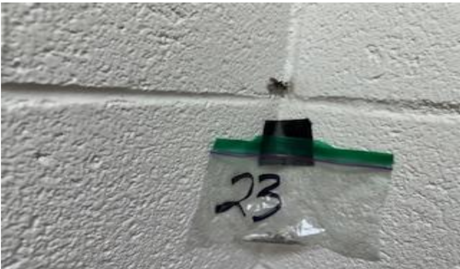
18. VIEW OF REPRESENTATIVE (TYPICAL) SAMPLE OF NON-ACM CMU AND MORTAR JOINT SEALANT LOCATED THROUGHOUT INTERIOR WALL SURFACES IN BUILDINGS AT THOMAS C. MARSH PREPARATORY ACADEMY
