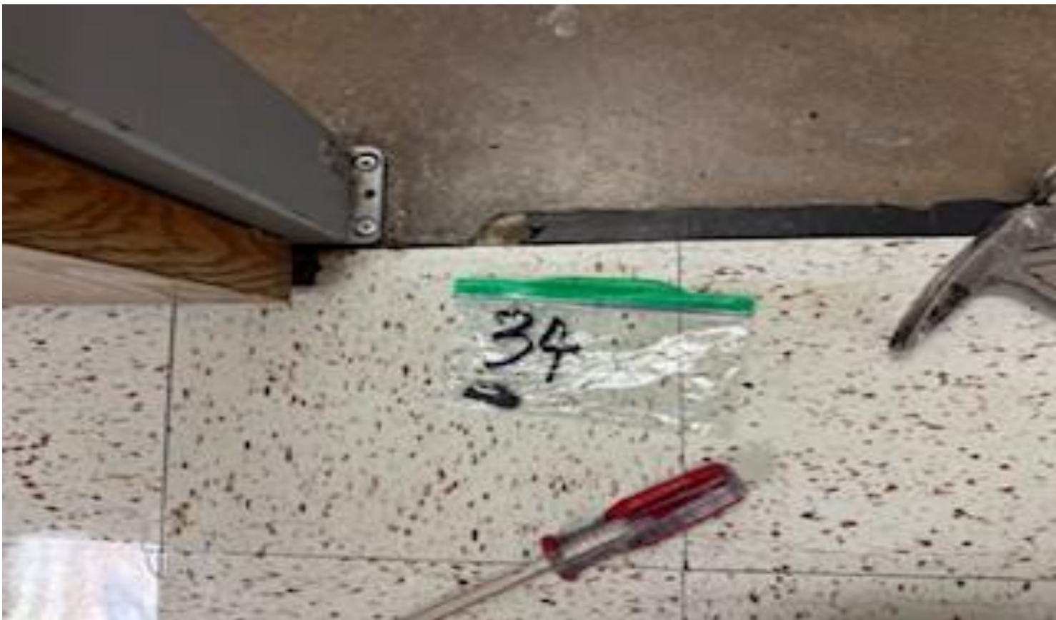
24. VIEW OF MORE REPRESENTATIVE (TYPICAL) SAMPLE OF ACM BLACK TRANSITION DOOR MASTIC AND SEALANT LOCATED AT DOOR ENTRANCES IN VARIOUS AREAS IN THE BUILDINGS AT THOMAS C. MARSH PREPARATORY ACADEMY
