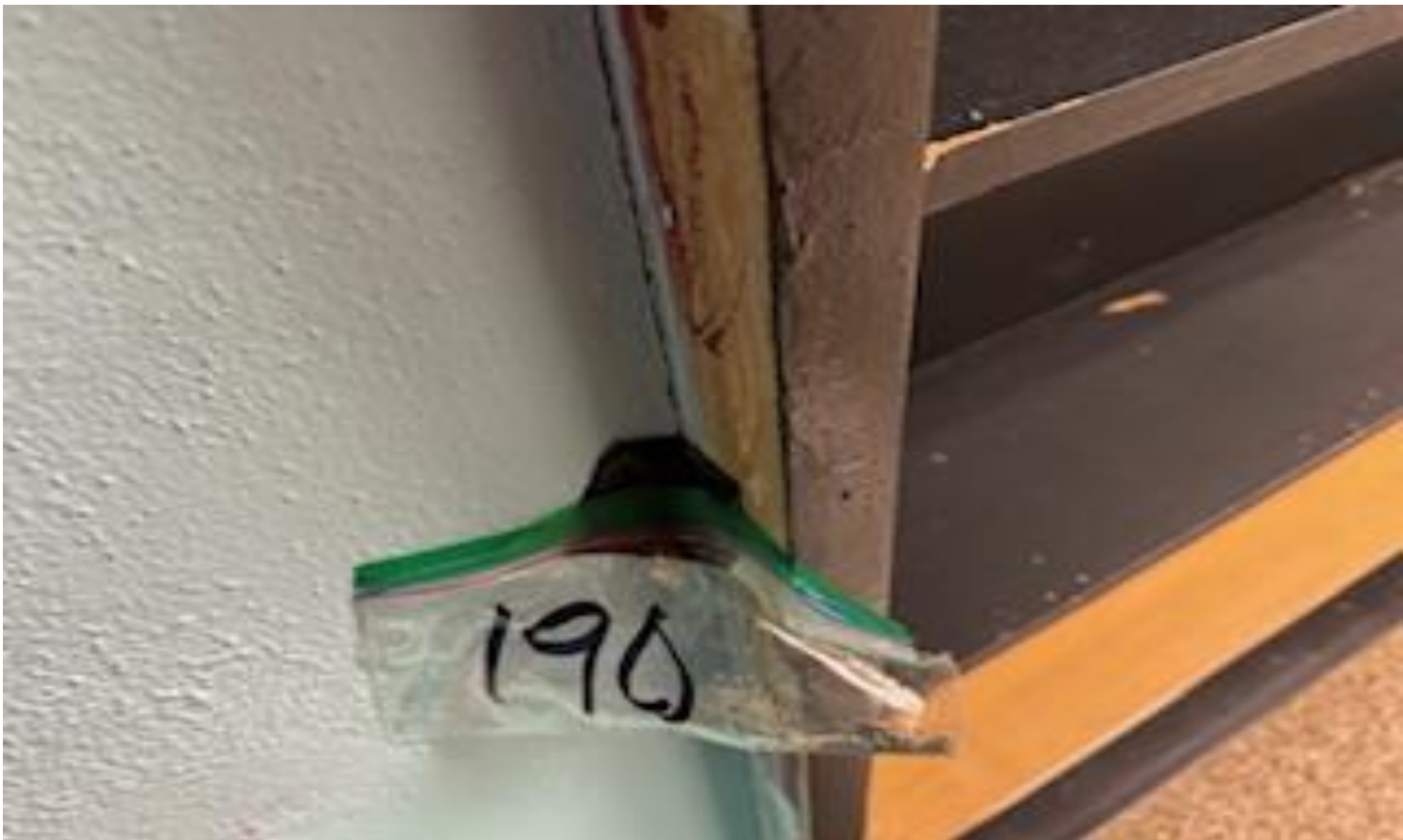
74. VIEW OF REPRESENTATIVE (TYPICAL) SAMPLE OF ACM CABINET WORKS CAULKING LOCATED THROUGHOUT CLASS ROOMS ON THE 3 RD FLOOR WALL SURFACES IN BUILDINGS AT THOMAS C. MARSH PREPARATORY ACADEMY
