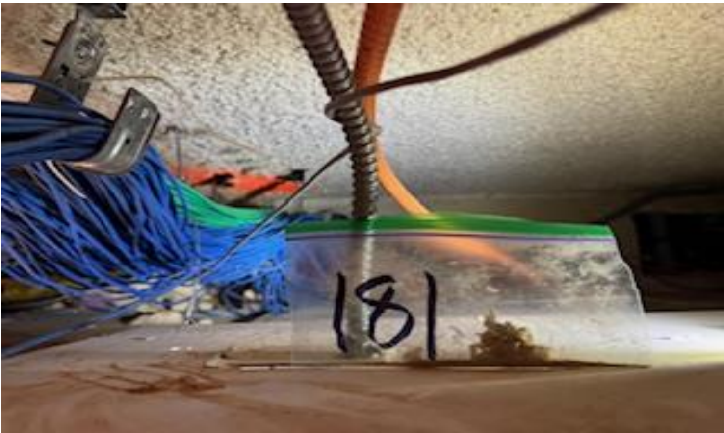
73 VIEW OF MORE REPRESENTATIVE (TYPICAL) SAMPLE OF ACM SPRAY-APPLIED CEILING (SAC) TEXTURE LOCATED ON INTERIOR 3 RD FLOOR CEILING IN BUILDING AT THOMAS C. MARSH PREPARATORY ACADEMY
