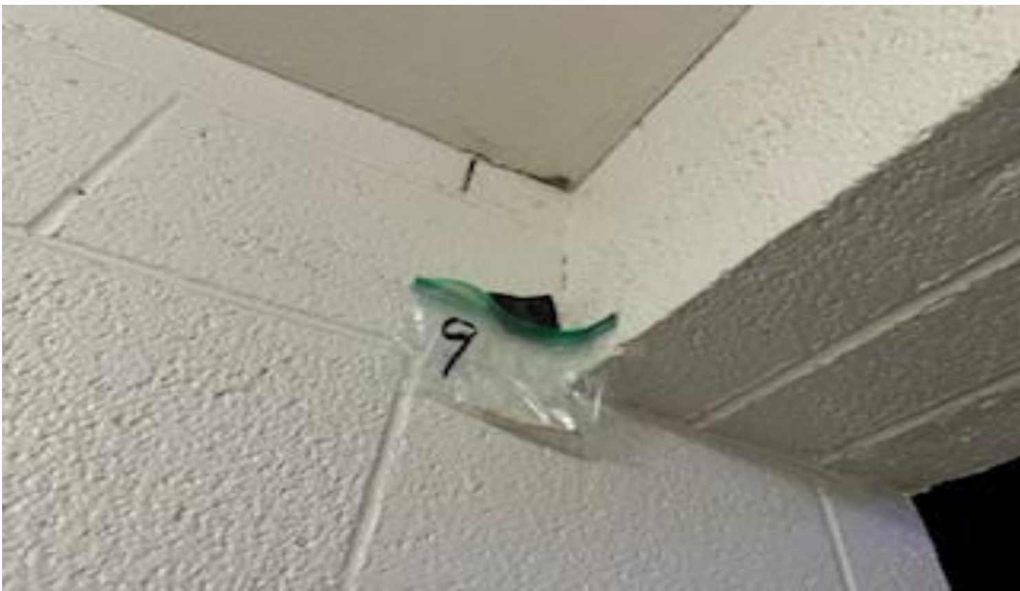
7. VIEW OF REPRESENTATIVE (TYPICAL) SAMPLE OF NON-ACM PLASTER CEILING LOCATED THROUGHOUT INTERIOR CEILING SURFACES IN BUILDINGS AT THOMAS C. MARSH PREPARATORY ACADEMY
