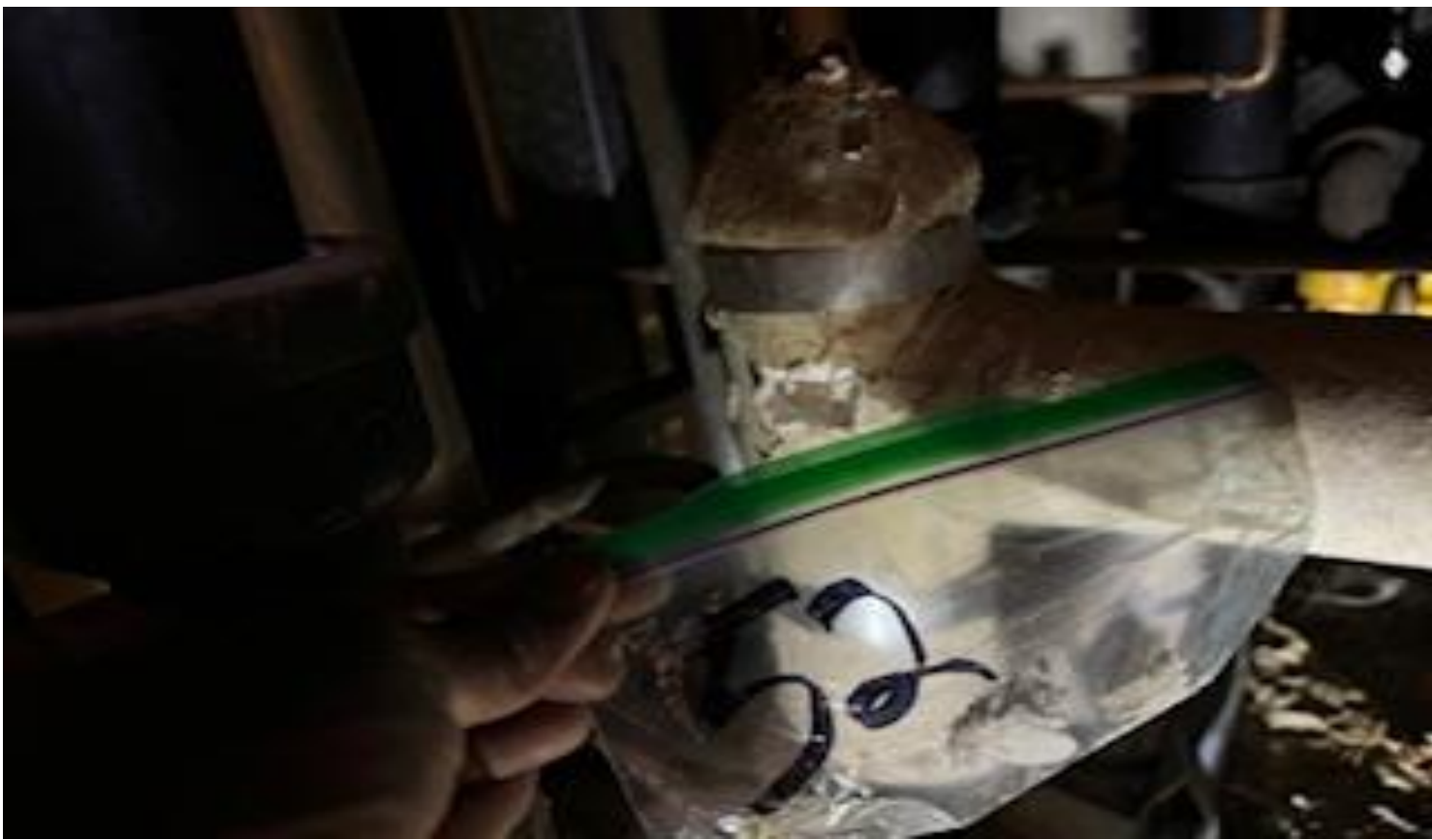
35. VIEW OF REPRESENTATIVE (TYPICAL) SAMPLE OF ACM THERMAL SYSTEMS INSULATION (TSI) ON T-FITTINGS LOCATED IN SOME AREAS IN BUILDINGS AT THOMAS C. MARSH PREPARATORY ACADEMY
