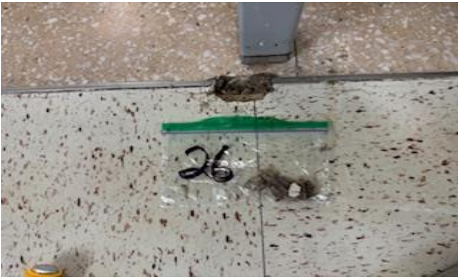
19. VIEW OF REPRESENTATION (TYPICAL) SAMPLE OF NON-ACM UNDER-LAYER FLOOR FLOAT LOCATED THROUGHOUT INTERIOR HALLWAY FLOORS IN BUILDINGS AT THOMAS C. MARSH PREPARATORY ACADEMY
