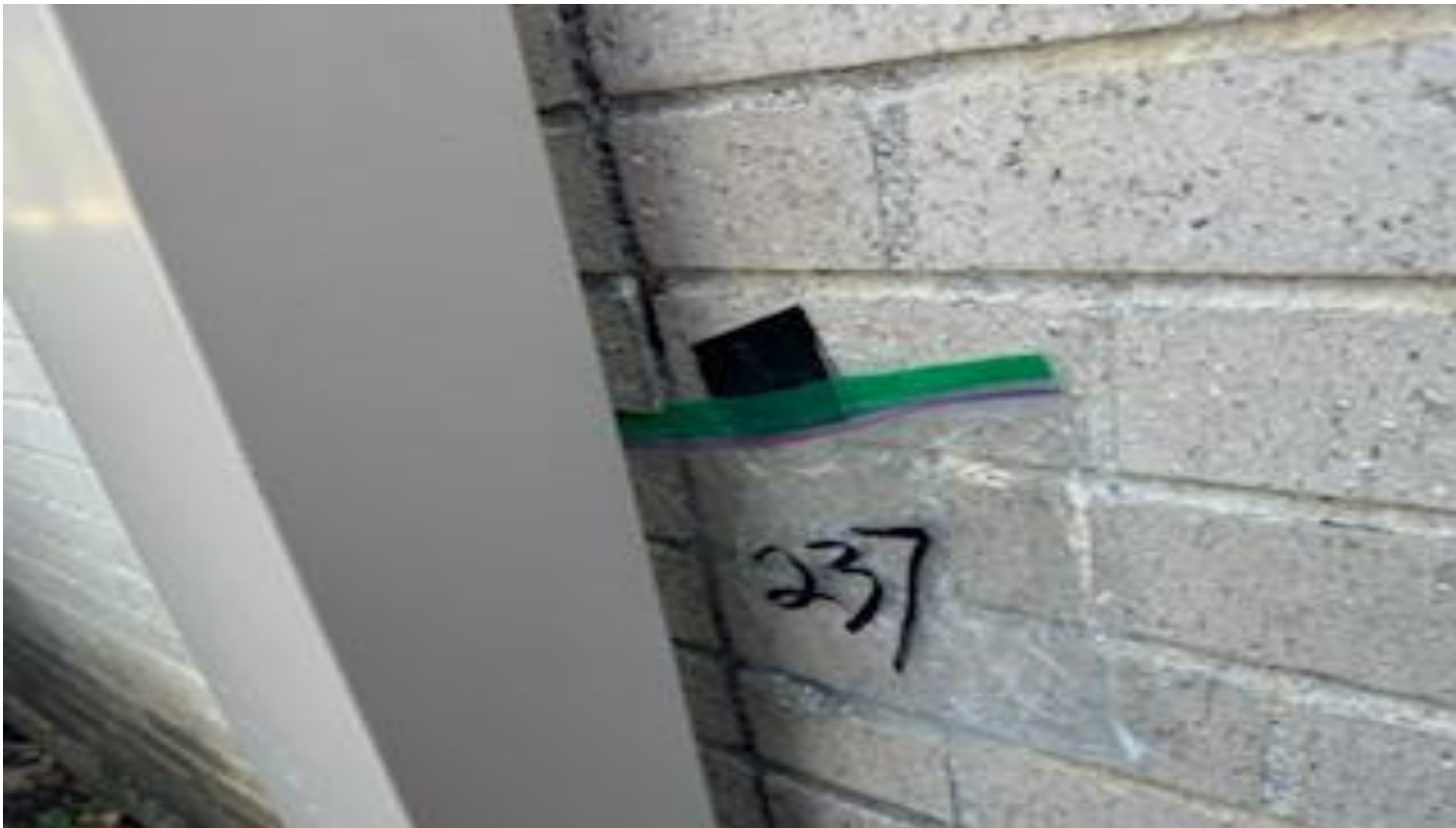
86. VIEW OF MORE REPRESENTATIVE (TYPICAL) SAMPLE OF ACM EXTERIOR BUILDING SEALANT LOCATED AT EXTERIOR BUILDING PENETRATIONS THROUGHOUT THE BUILDINGS AT THOMAS C. MARSH PREPARATORY ACADEMY
