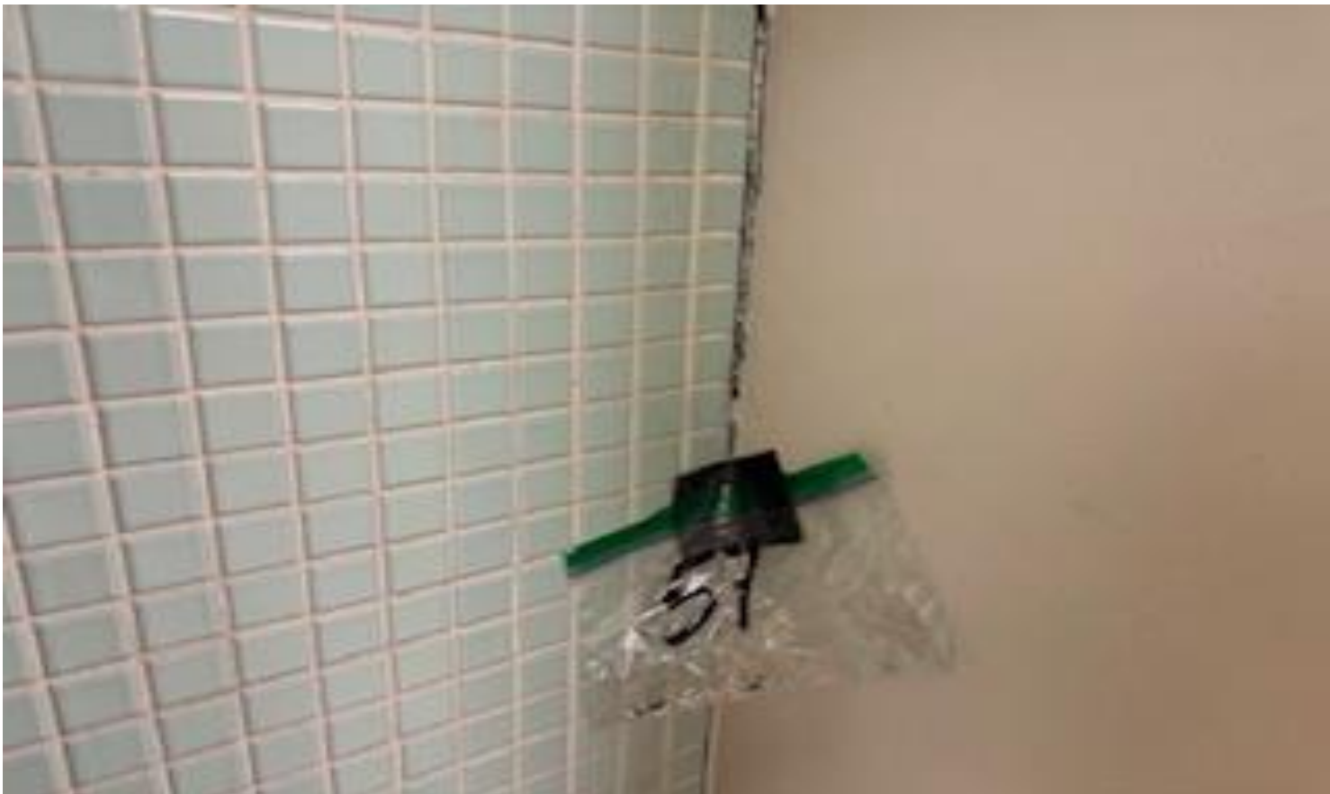
40. VIEW OF REPRESENTATIVE (TYPICAL) SAMPLE OF NON-ACM STUDENT LOCKERS CAULKING LOCATED THROUGHOUT THE HALLWAYS IN BUILDINGS AT THOMAS C. MARSH PREPARATORY ACADEMY
