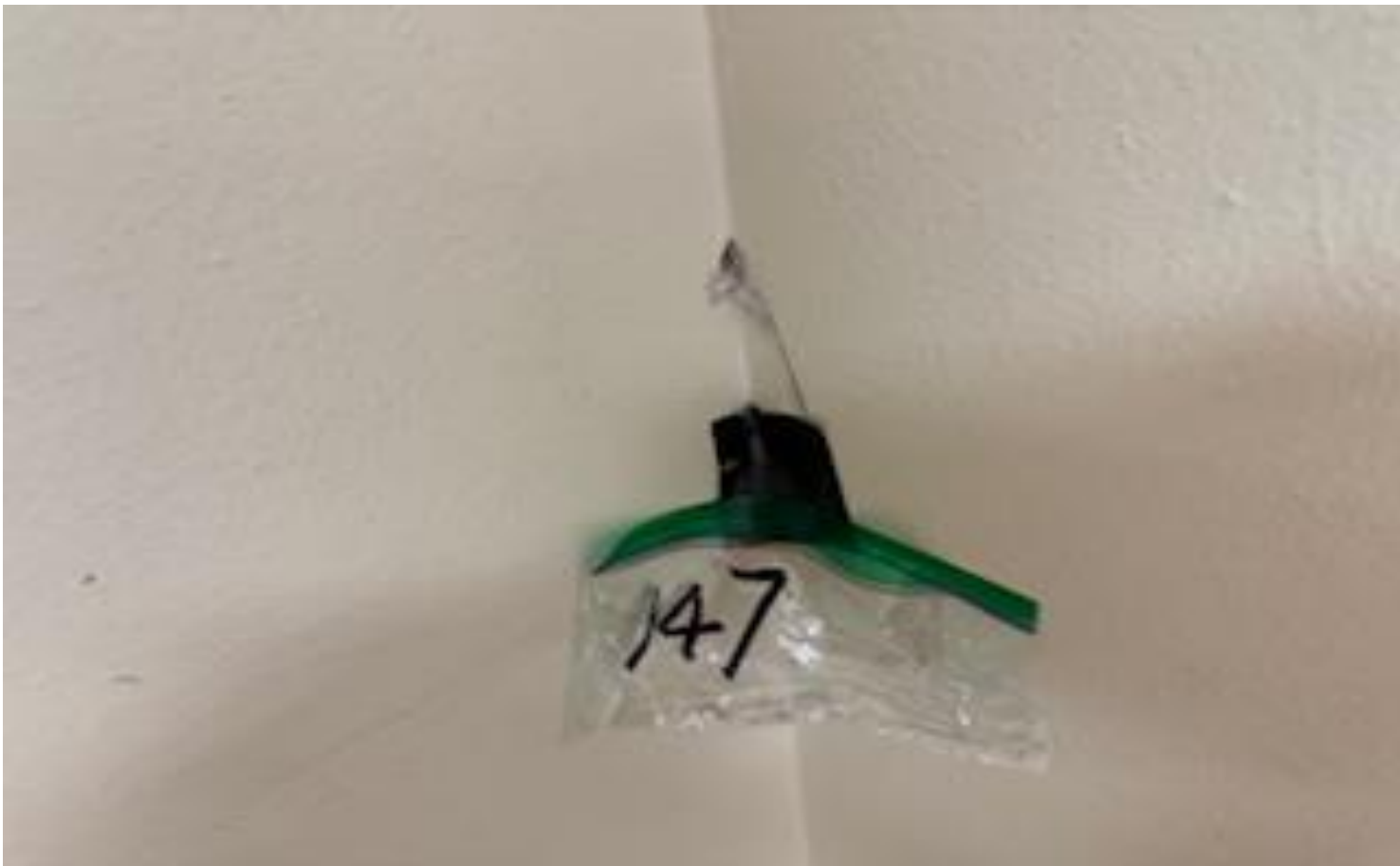
64. VIEW OF REPRESENTATIVE (TYPICAL) SAMPLE OF NON-ACM WALL TEXTURE JOINT COMPOUND AND SHEETROCK MUD LOCATED IN SEVERAL AREAS THROUGHOUT THE BUILDINGS AT THOMAS C. MARSH PREPARATORY ACADEMY
