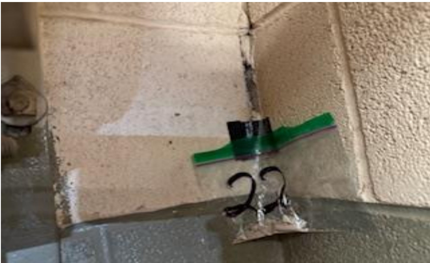
17. VIEW OF REPRESENTATIVE (TYPICAL) SAMPLE OF NON-ACM CONCRETE MASONRY UNITS (CMU) AND MORTAR LOCATED THROUGHOUT INTERIOR WALL SURFACES IN BUILDINGS AT THOMAS C. MARSH PREPARATORY ACADEMY
