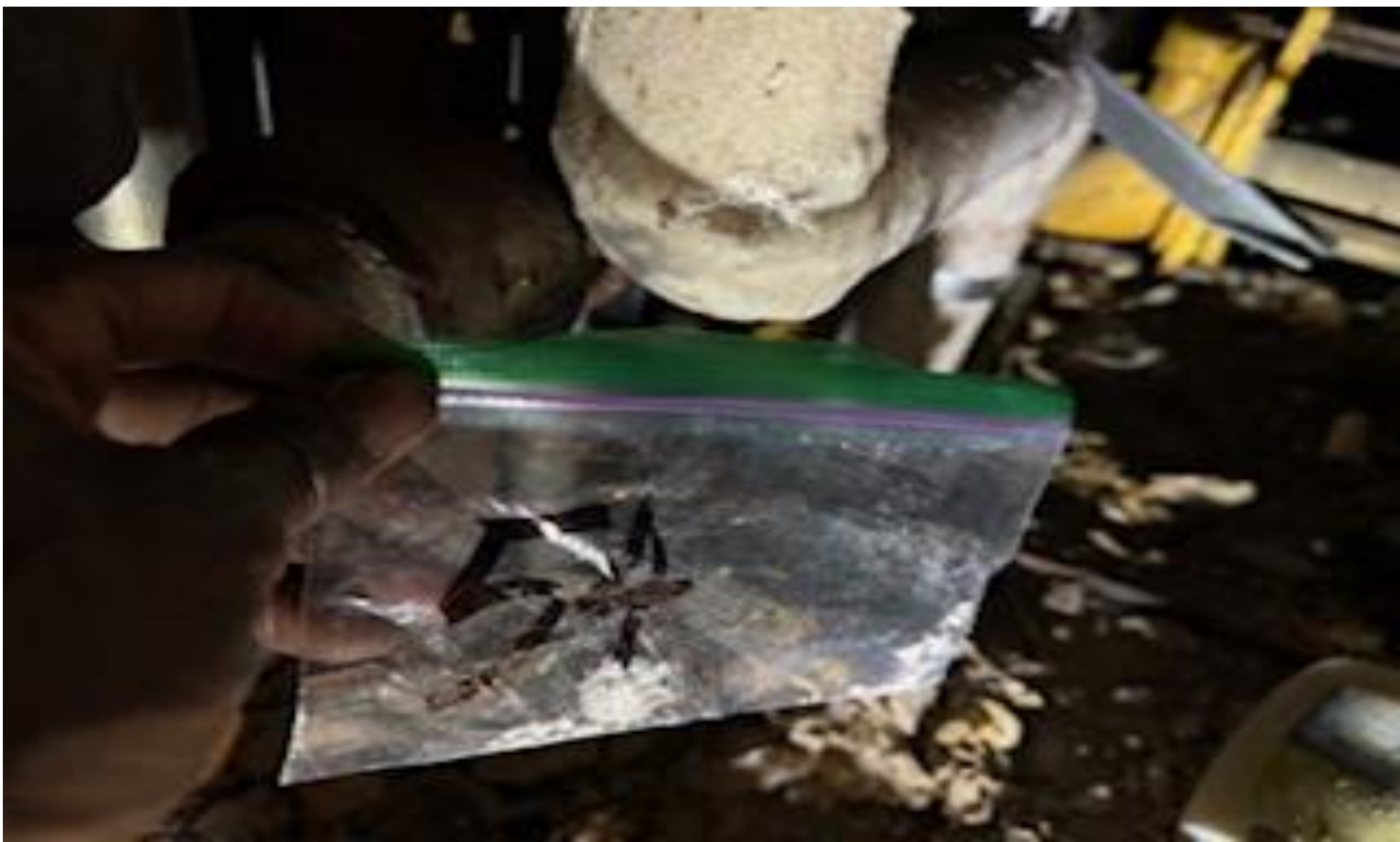
37. VIEW OF MORE REPRESENTATIVE (TYPICAL) SAMPLE OF ACM THERMAL SYSTEMS INSULATION (TSI) ON ELBOWS LOCATED IN SOME AREAS IN BUILDINGS AT THOMAS C. MARSH PREPARATORY ACADEMY
