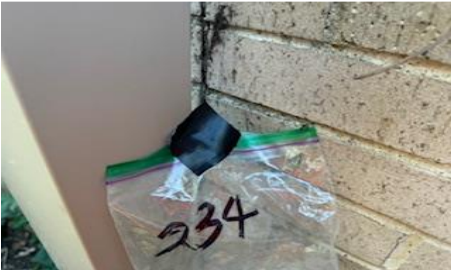
86. VIEW OF REPRESENTATIVE (TYPICAL) SAMPLE OF ACM EXTERIOR BUILDING SEALANT LOCATED AT EXTERIOR BUILDING PENETRATIONS THROUGHOUT THE BUILDINGS AT THOMAS C. MARSH PREPARATORY ACADEMY
