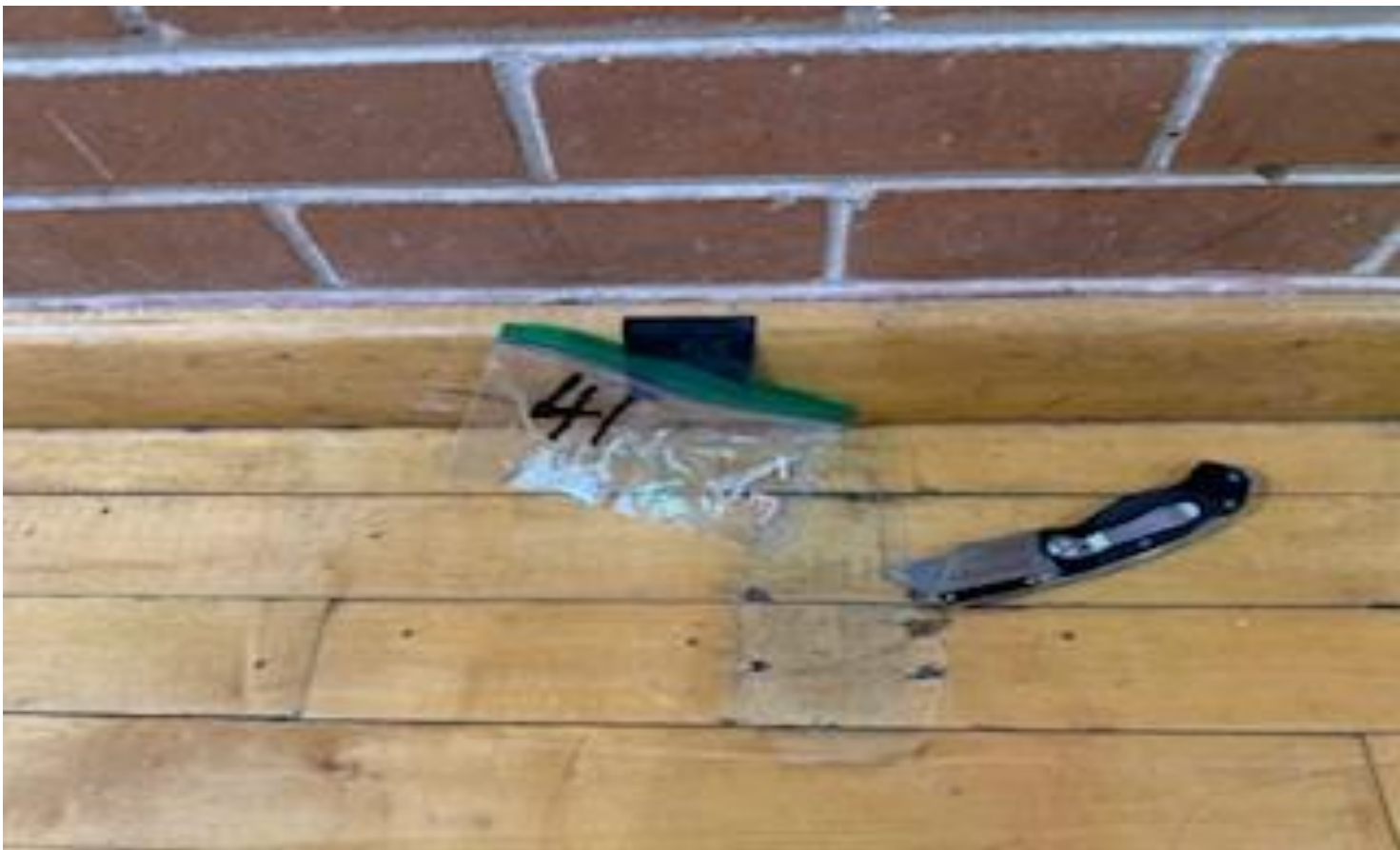
30. VIEW OF REPRESENTATIVE (TYPICAL) SAMPLE OF ACM WOOD COVE-BASE CAULKING AND SEALANT LOCATED IN BASKET BALL COURTS AND ELSEWHERE IN BUILDINGS AT THOMAS C. MARSH PREPARATORY ACADEMY
