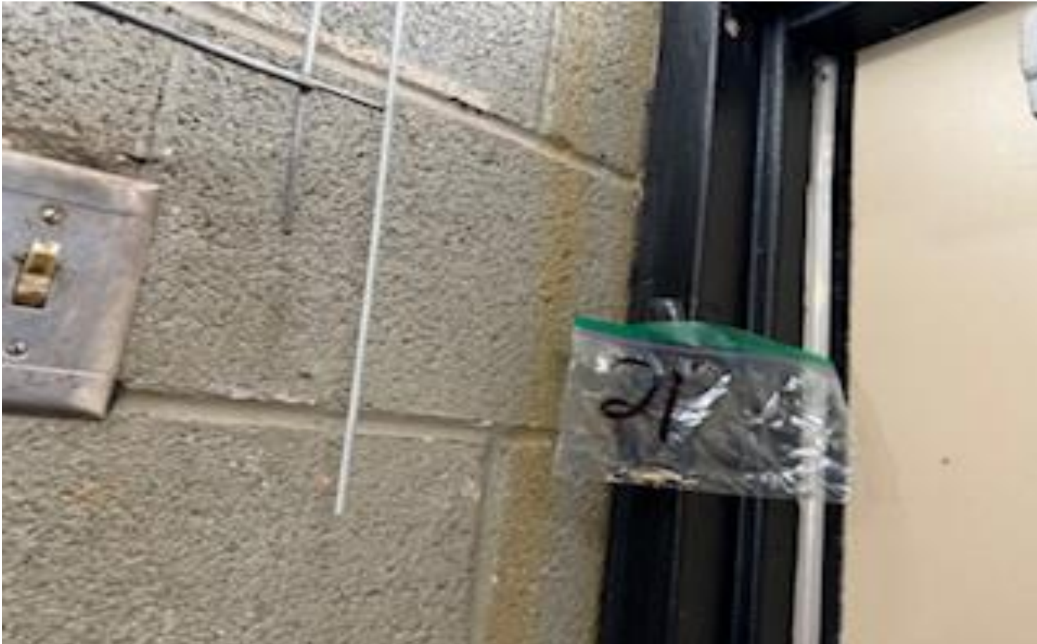
16. VIEW OF REPRESENTATIVE (TYPICAL) SAMPLE OF ACM DOOR CAULKING LOCATED THROUGHOUT INTERIOR DOOR FRAMES IN BUILDINGS AT THOMAS C. MARSH PREPARATORY ACADEMY
