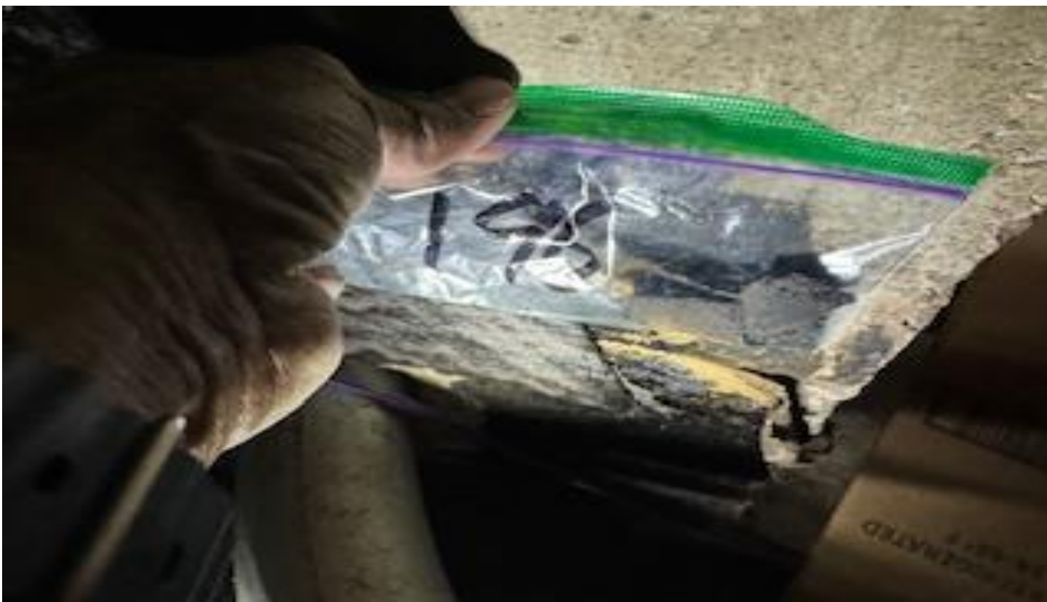
78. VIEW OF REPRESENTATIVE (TYPICAL) SAMPLE OF ACM THERMAL WALL INSULATION LOCATED ON PERIMETER WALLS IN THE CRAWL SPACE UNDERNEATH ALL BUILDINGS AT THOMAS C. MARSH PREPARATORY ACADEMY
