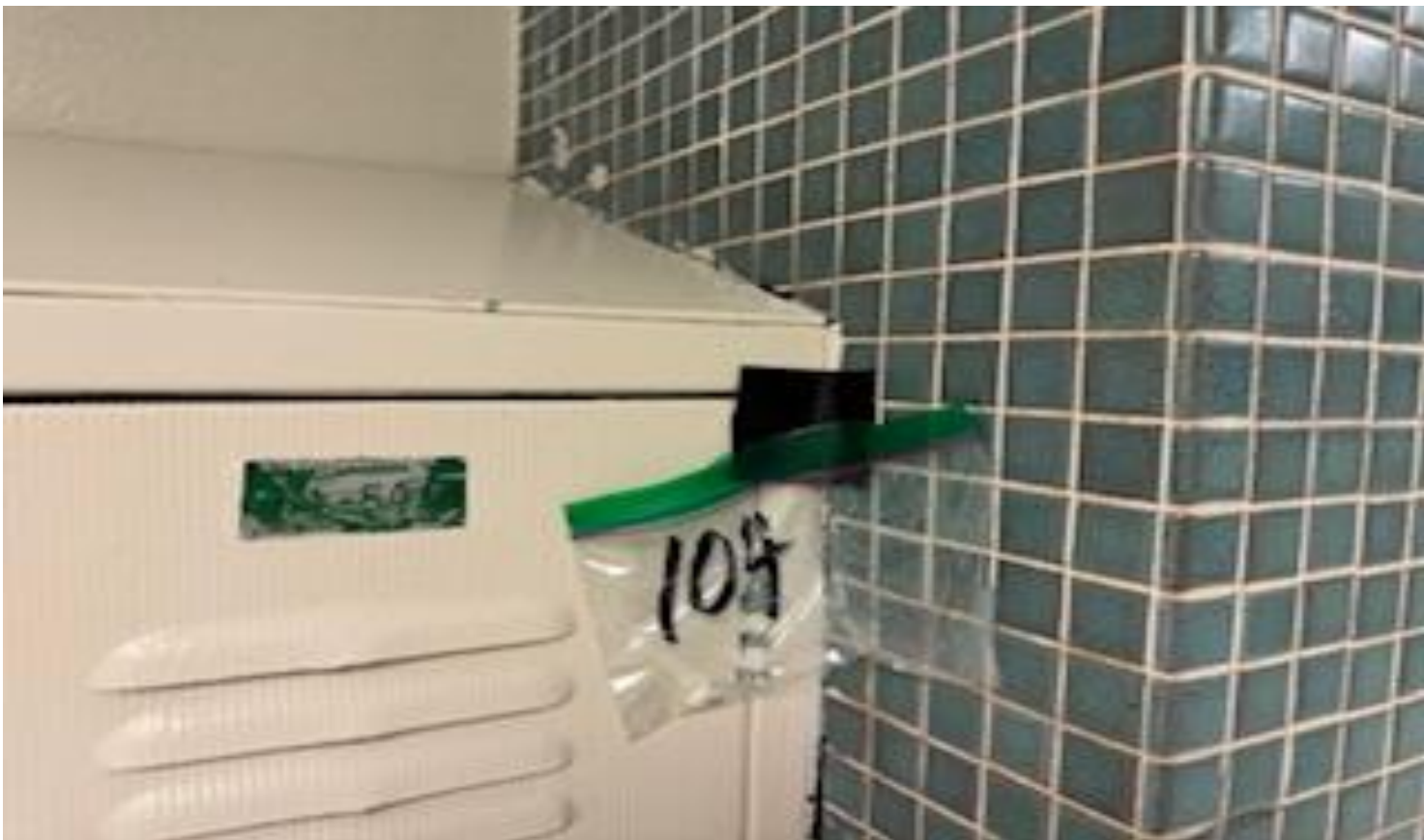
52 VIEW OF MORE REPRESENTATIVE (TYPICAL) SAMPLE OF NON-ACM STUDENT LOCKERS CAULKING LOCATED THROUGHOUT THE HALLWAYS IN BUILDINGS AT THOMAS C. MARSH PREPARATORY ACADEMY
