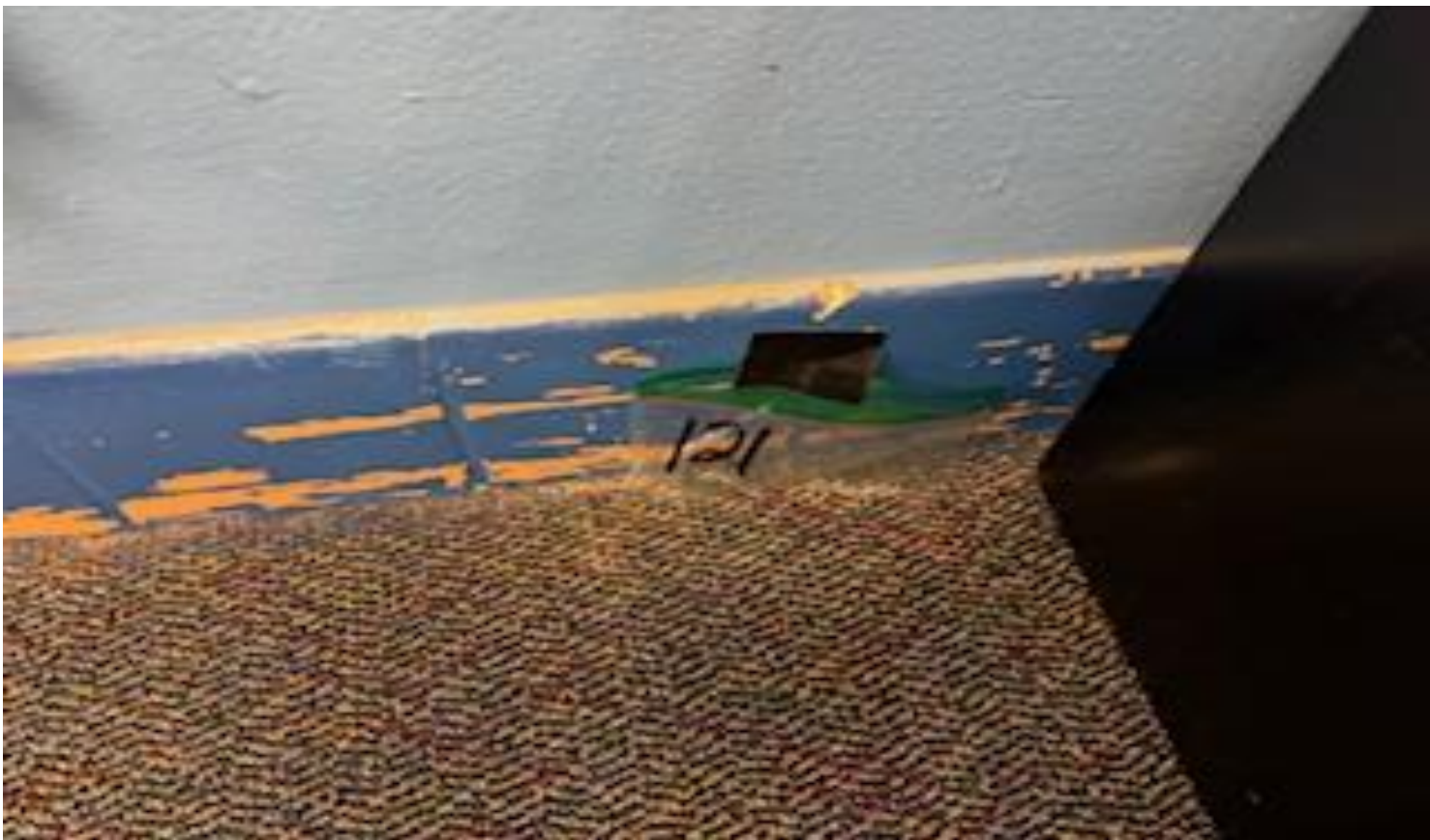
56. VIEW OF MORE REPRESENTATIVE (TYPICAL) SAMPLE OF NON-ACM COVE-BASE CERAMIC TILES AND GROUT LOCATED THROUGHOUT THE BUILDINGS AT THOMAS C. MARSH PREPARATORY ACADEMY
