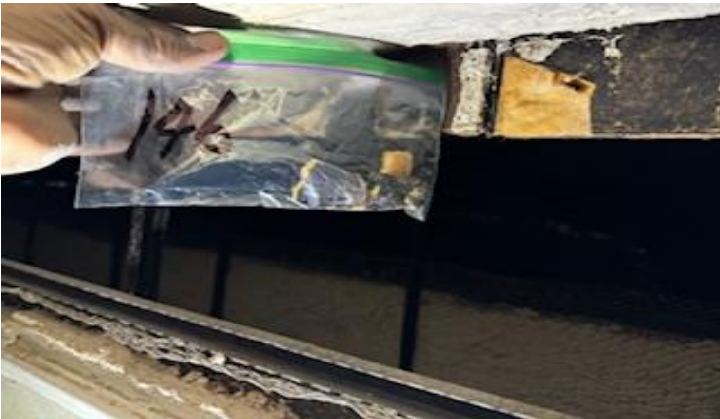
63. VIEW OF REPRESENTATIVE (TYPICAL) SAMPLE OF NON-ACM BLACK MASTIC ON FOAM INSULATION LOCATED ABOVE CEILING ON THE 2 ND FLOOR IN A BUILDING AT THE THOMAS C. MARSH PREPARATORY ACADEMY
