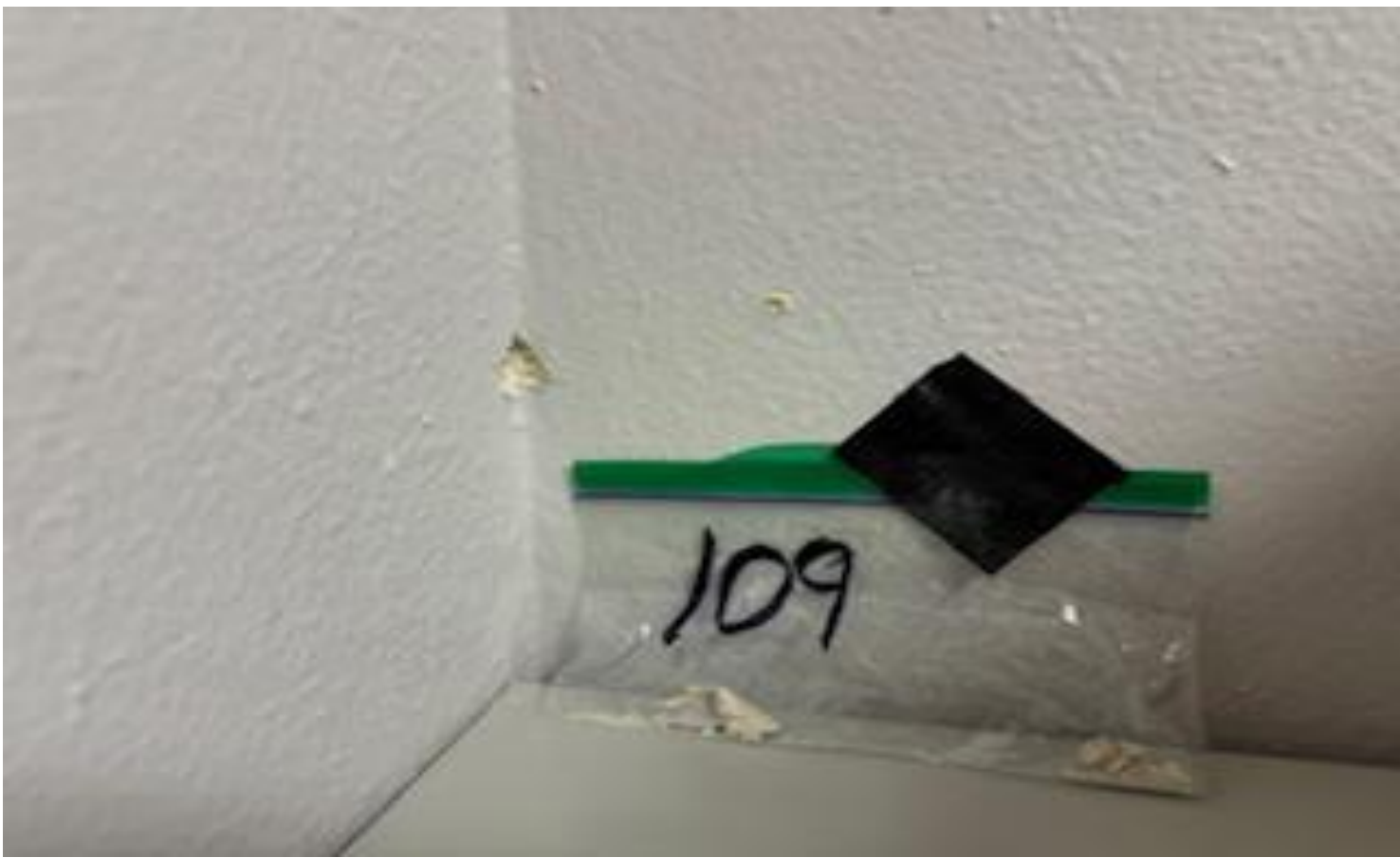
53 VIEW OF REPRESENTATIVE (TYPICAL) SAMPLE OF ACM WALL TEXTURE JOINT COMPOUND AND SHEETROCK MUD LOCATED IN THE EXECUTIVE SUITE 118 IN A BUILDING AT THOMAS C. MARSH PREPARATORY ACADEMY
