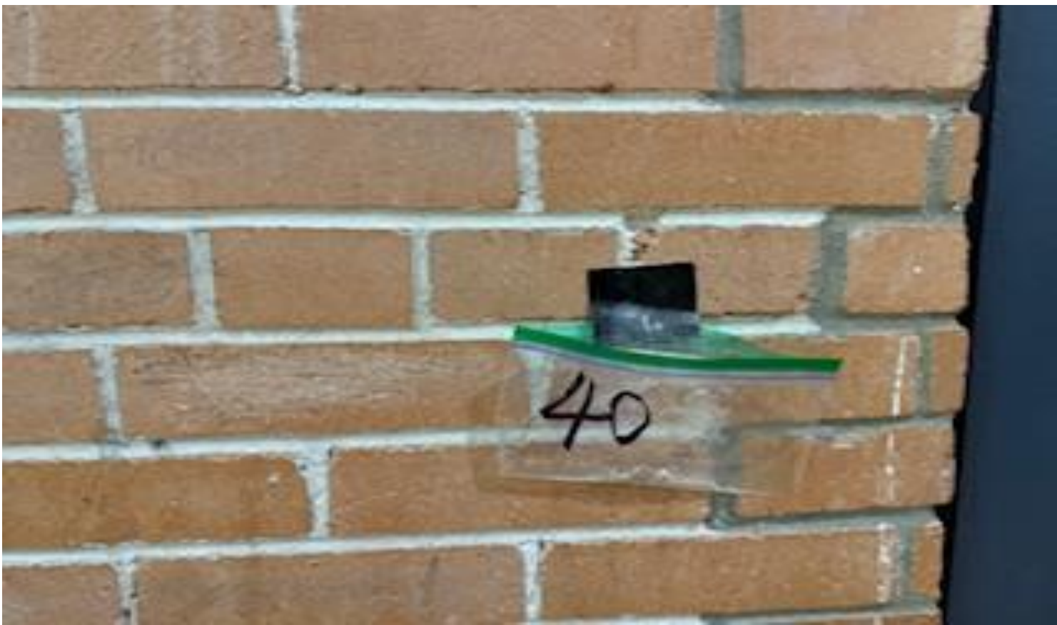
29. VIEW OF MORE REPRESENTATIVE (TYPICAL) SAMPLE OF NON-ACM INTERIOR BRICK AND MORTAR LOCATED IN VARIOUS AREAS THROUGHOUT THE BUILDINGS AT THOMAS C. MARSH PREPARATORY ACADEMY
