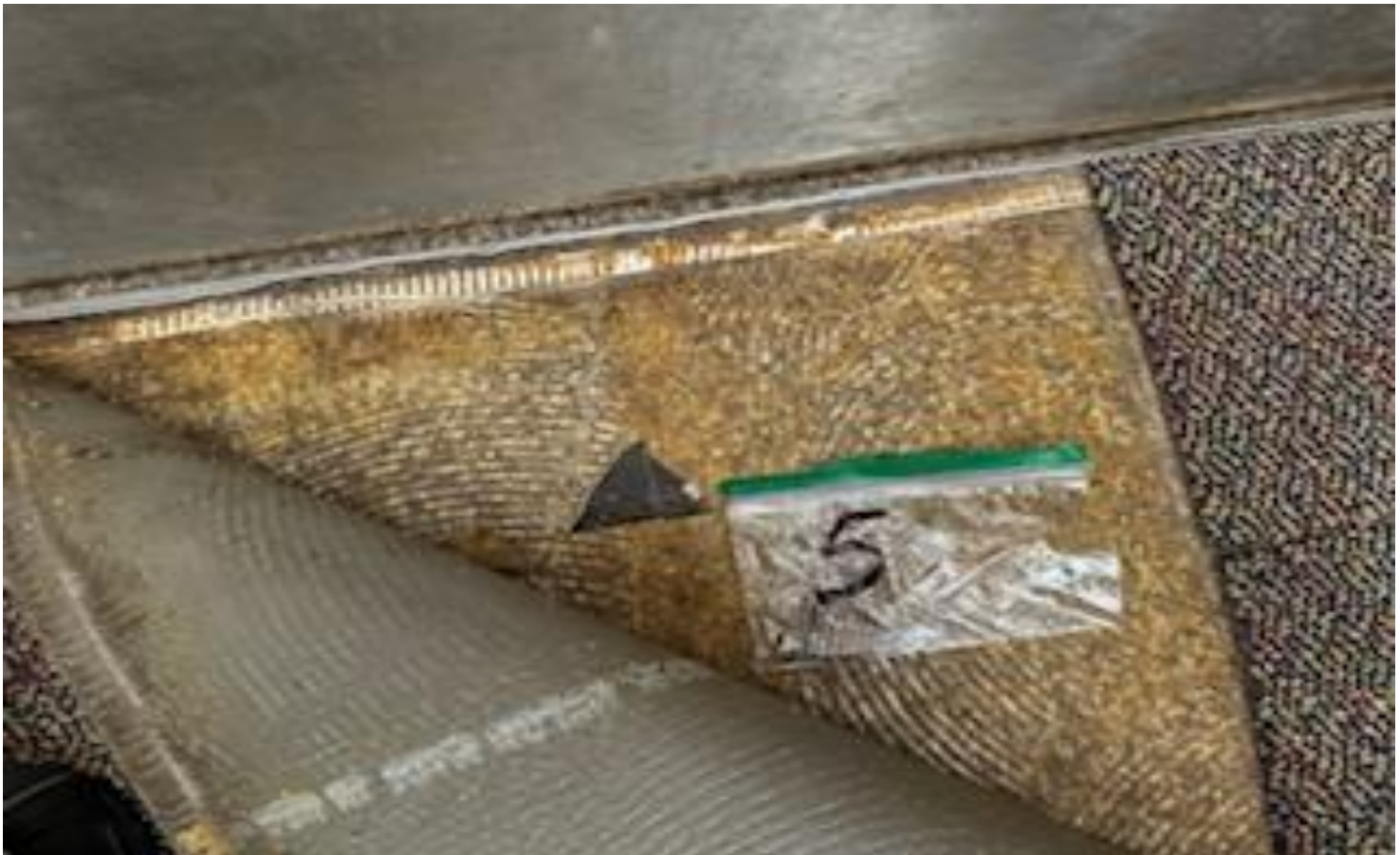
4. VIEW OF REPRESENTATIVE (TYPICAL) SAMPLE OF ACM DARK BROWN 9" X 9" FLOOR TILES AND BLACK MASTIC LOCATED IN VARIOUS AREAS THROUGHOUT INTERIOR FLOORS IN BUILDINGS AT THOMAS C. MARSH PREPARATORY ACADEMY
