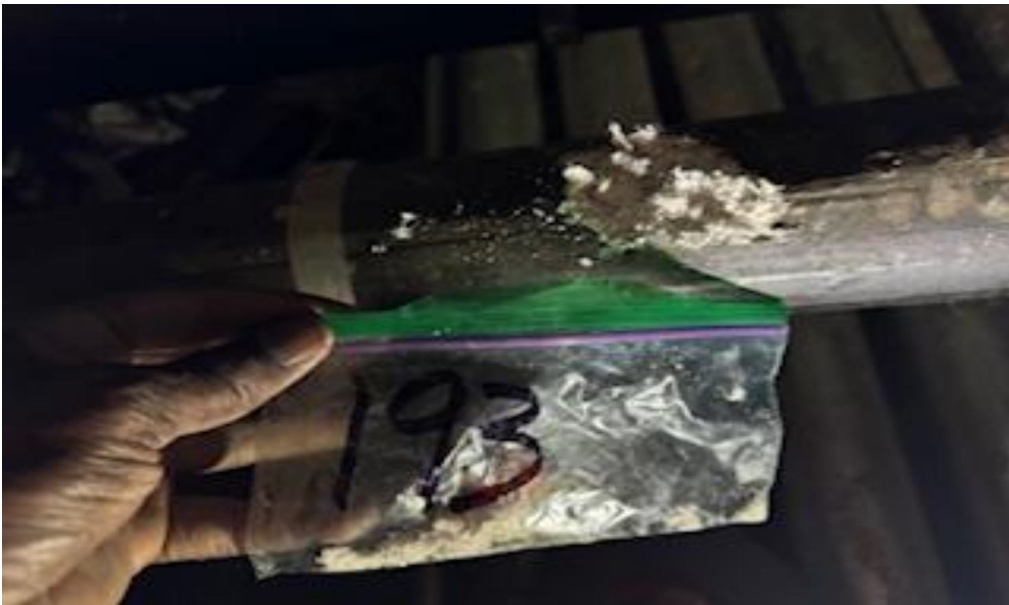
76. VIEW OF MORE REPRESENTATIVE (TYPICAL) SAMPLE OF ACM THERMAL SYSTEMS INSULATION (TSI) ON T-FITTINGS LOCATED IN THE CRAWL SPACE UNDERNEATH ALL BUILDINGS AT THOMAS C. MARSH PREPARATORY ACADEMY
