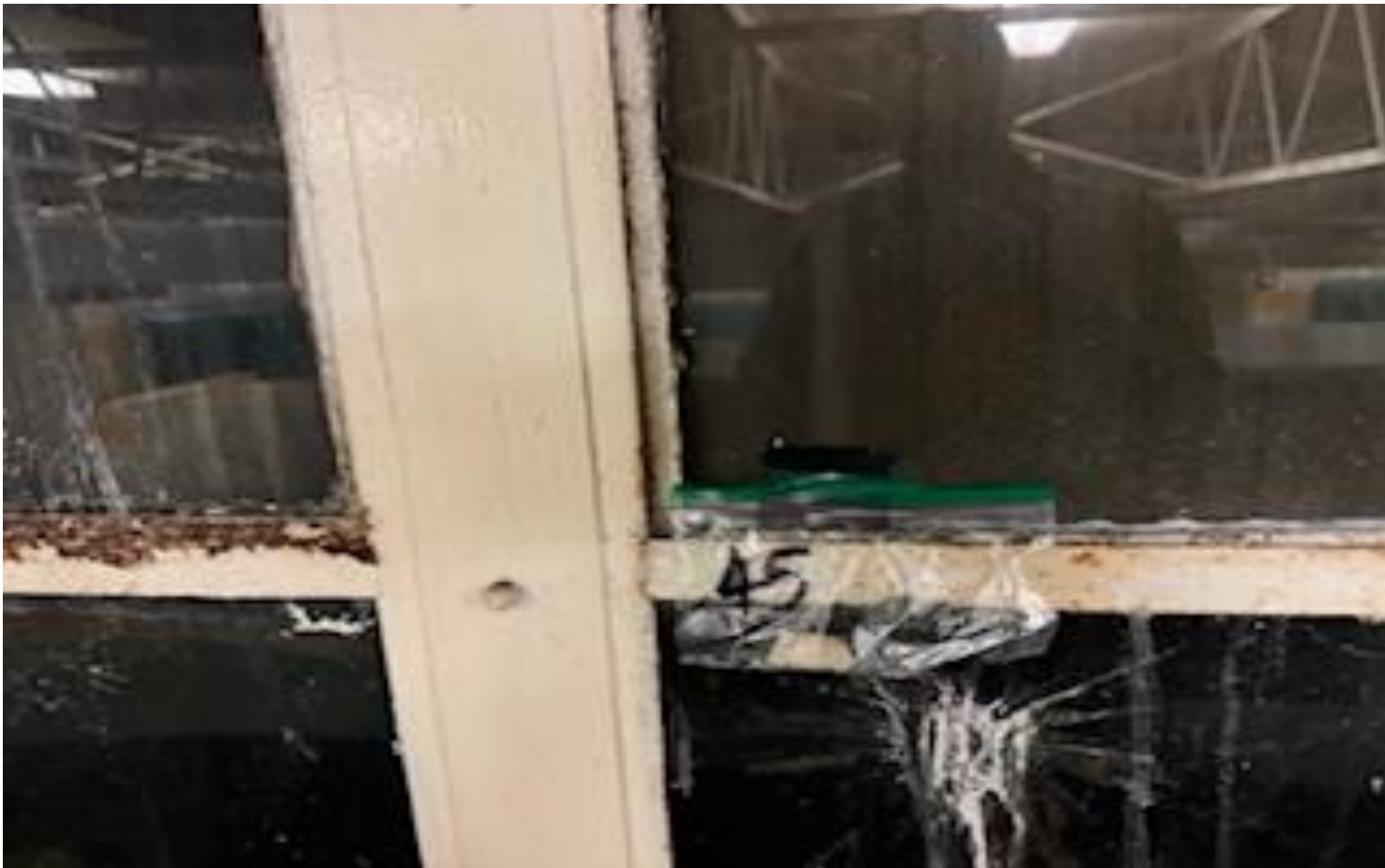
32. VIEW OF MORE REPRESENTATIVE (TYPICAL) SAMPLE OF ACM INTERIOR WINDOW GLASS PANES CAULKING LOCATED THROUGHOUT THE BUILDINGS AT THOMAS C. MARSH PREPARATORY ACADEMY
