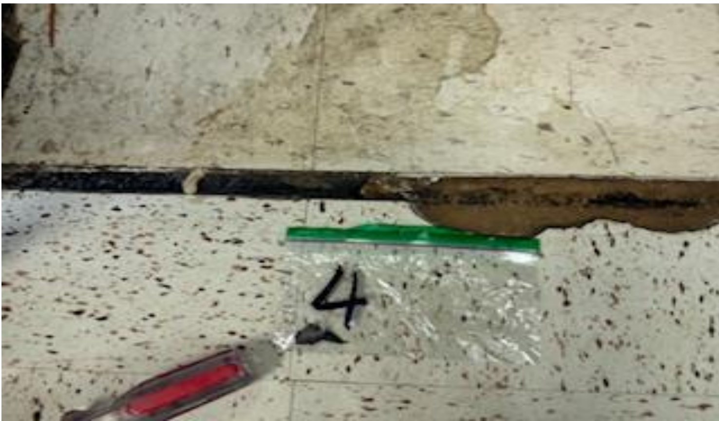
3. VIEW OF REPRESENTATIVE (TYPICAL) SAMPLE OF ACM BLACK TRANSITION DOOR MASTIC AND SEALANT LOCATED AT DOOR ENTRANCES IN VARIOUS AREAS IN THE BUILDINGS AT THOMAS C. MARSH PREPARATORY ACADEMY
