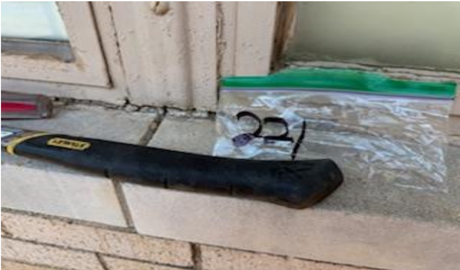
84. VIEW OF REPRESENTATIVE (TYPICAL) SAMPLE OF ACM EXTERIOR WINDOW CAULKING LOCATED ON EXTERIOR WINDOW FRAMES THROUGHOUT THE BUILDING AT THOMAS C. MARSH PREPARATORY ACADEMY
