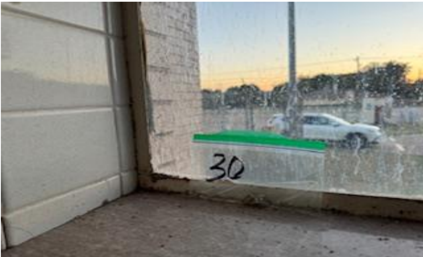
22. VIEW OF MORE REPRESENTATIVE (TYPICAL) SAMPLE OF ACM WINDOW CAULKING LOCATED THROUGHOUT INTERIOR WINDOW FRAMES IN BUILDINGS AT THOMAS C. MARSH PREPARATORY ACADEMY
