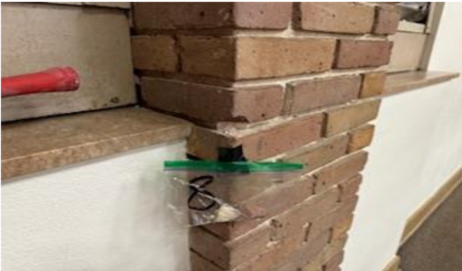
6. VIEW OF REPRESENTATIVE (TYPICAL) SAMPLE OF NON-ACM INTERIOR BRICK AND MORTAR LOCATED IN VARIOUS AREAS THROUGHOUT THE BUILDINGS AT THOMAS C. MARSH PREPARATORY ACADEMY
