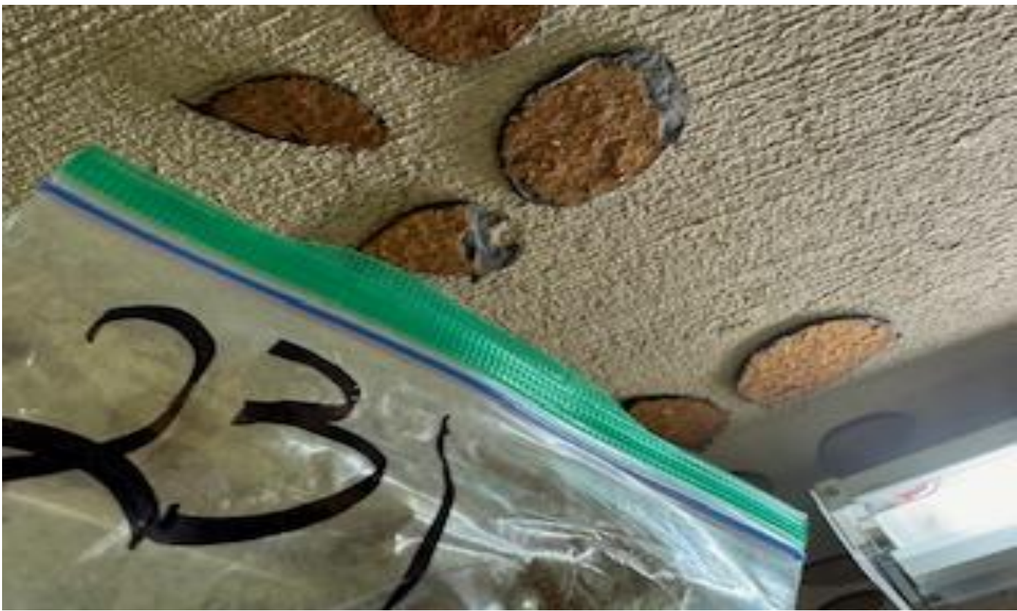
85. VIEW OF REPRESENTATIVE (TYPICAL) SAMPLE OF ACM 1' X 1' STOCK-ON CEILING TILES AND DOT MASTIC LOCATED IN SOME AREAS IN BUILDINGS AT THOMAS C. MARSH PREPARATORY ACADEMY
