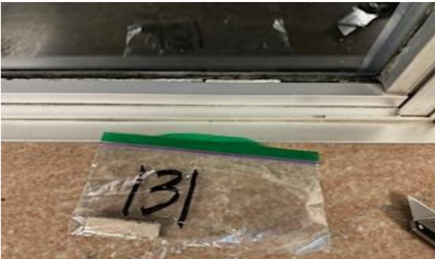
59. VIEW OF REPRESENTATIVE (TYPICAL) SAMPLE OF ACM INTERIOR WINDOW CAULKING LOCATED THROUGHOUT THE INTERIOR 2 ND FLOOR WALL SURFACES IN BUILDINGS AT THOMAS C. MARSH PREPARATORY ACADEMY
