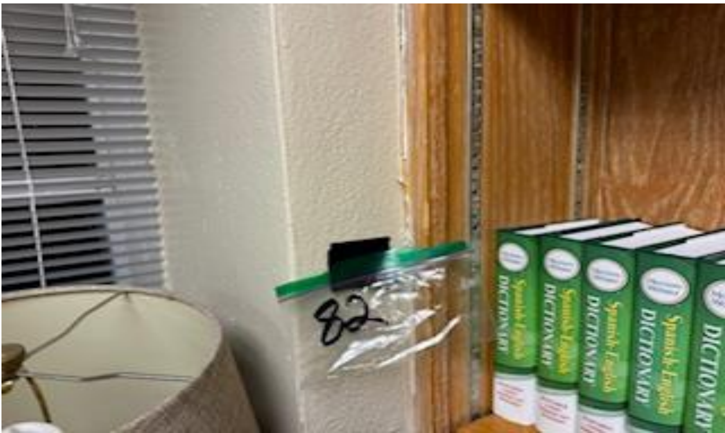
47 VIEW OF REPRESENTATIVE (TYPICAL) SAMPLE OF ACM CAULKING ON CABINET WORKS LOCATED IN CLASS ROOMS AND ELSEWHERE THROUGHOUT THE BUILDINGS AT THOMAS C. MARSH PREPARATORY ACADEMY
