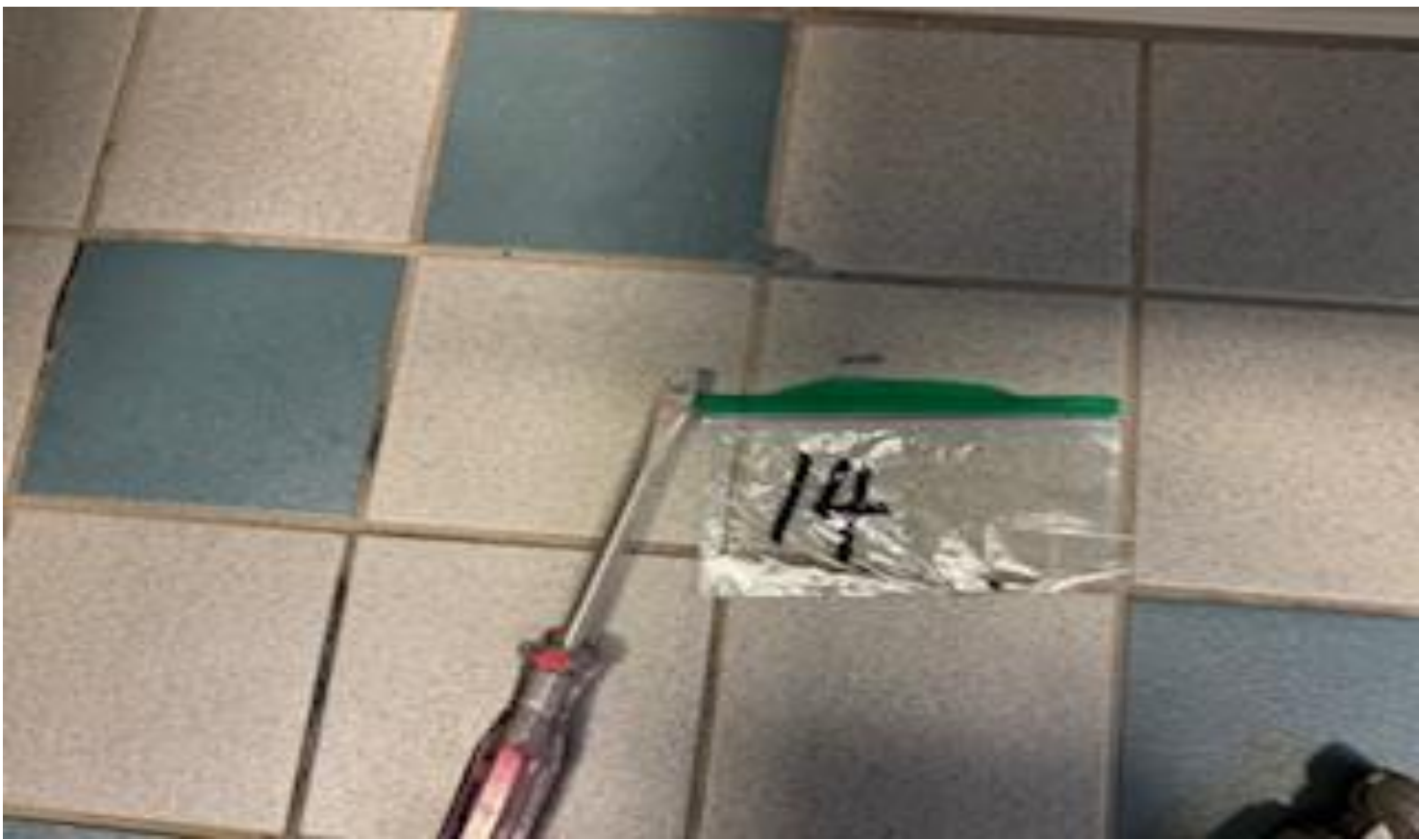
11. VIEW OF REPRESENTATIVE (TYPICAL) SAMPLE OF NON-ACM PATTERNED WALL CERAMIC TILES AND GROUT LOCATED IN VARIOUS WET AREAS THROUGHOUT THE BUILDINGS AT THOMAS C. MARSH PREPARATORY ACADEMY
