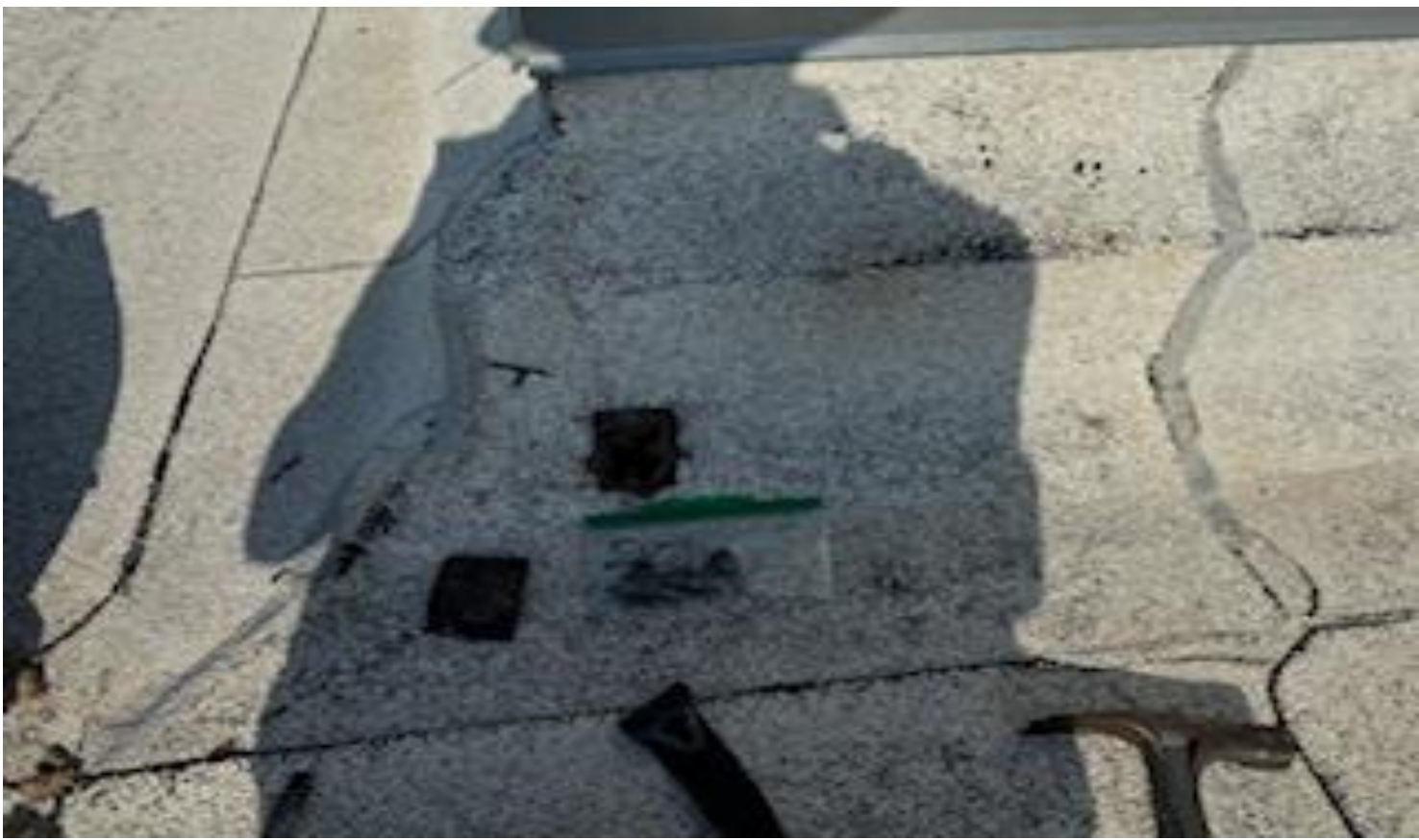
79. VIEW OF REPRESENTATIVE (TYPICAL) SAMPLE OF NON-ACM HVAC BASE MASTIC SEALANT LOCATED THROUGHOUT TOP ROOFS OF THE BUILDINGS AT THOMAS C. MARSH PREPARATORY ACADEMY
