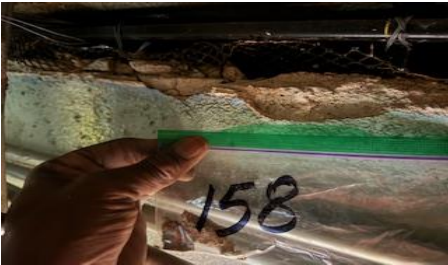
67. VIEW OF REPRESENTATIVE (TYPICAL) SAMPLE OF ACM SAC-CONTAMINATED PLASTER WALL LOCATED IN CLASS ROOM 215B ON THE 2 ND FLOOR IN A BUILDING AT THOMAS C. MARSH PREPARATORY ACADEMY
