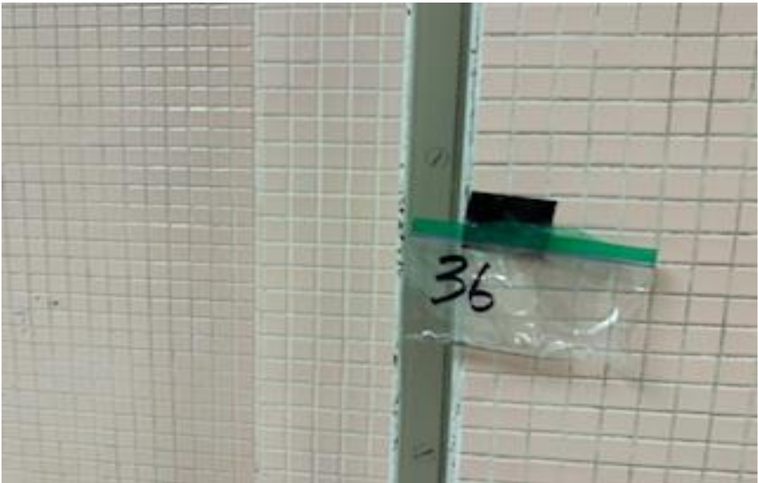
26. VIEW OF REPRESENTATIVE (TYPICAL) SAMPLE OF NON-ACM BUILDING DEMARCATION SEALANT LOCATED ON VARIOUS INTERIOR WALL SURFACES THROUGHOUT THE BUILDINGS AT THOMAS C. MARSH PREPARATORY ACADEMY
