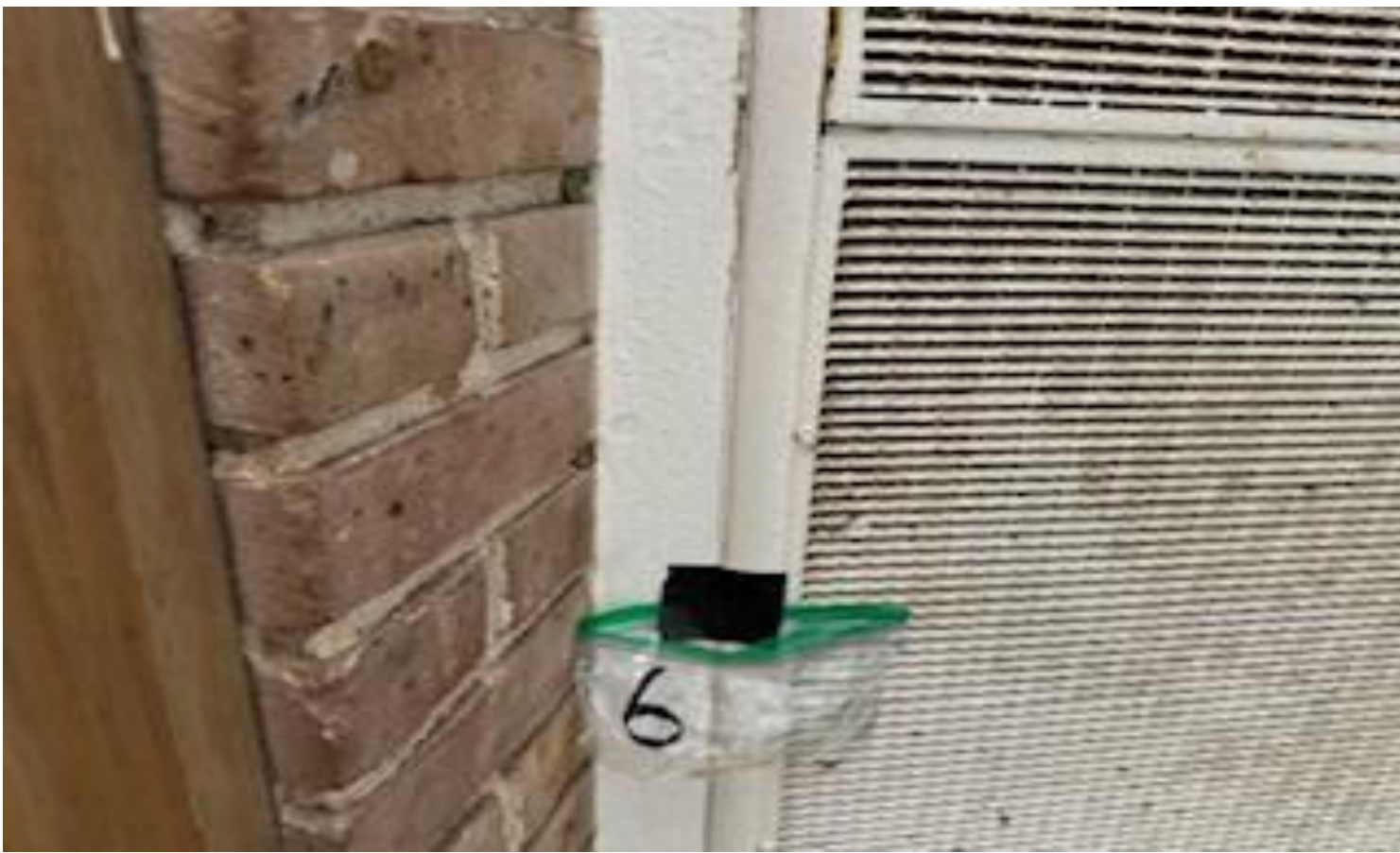
5. VIEW OF REPRESENTATIVE (TYPICAL) SAMPLE OF NON-ACM RETURN AIR-GRILL CAULKING LOCATED AT BACK ENTRANCE TO THE AUDITORIUM IN A BUILDING AT THOMAS C. MARSH PREPARATORY ACADEMY
