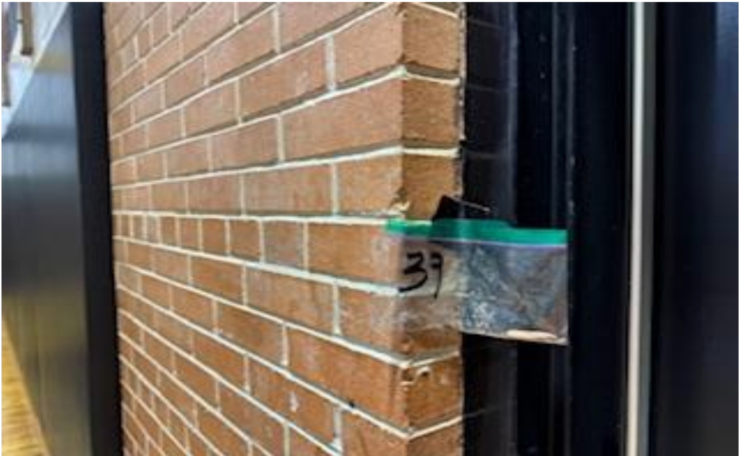
28. VIEW OF MORE REPRESENTATIVE (TYPICAL) SAMPLE OF ACM DOOR CAULKING LOCATED THROUGHOUT INTERIOR DOOR FRAMES IN BUILDINGS AT THOMAS C. MARSH PREPARATORY ACADEMY
