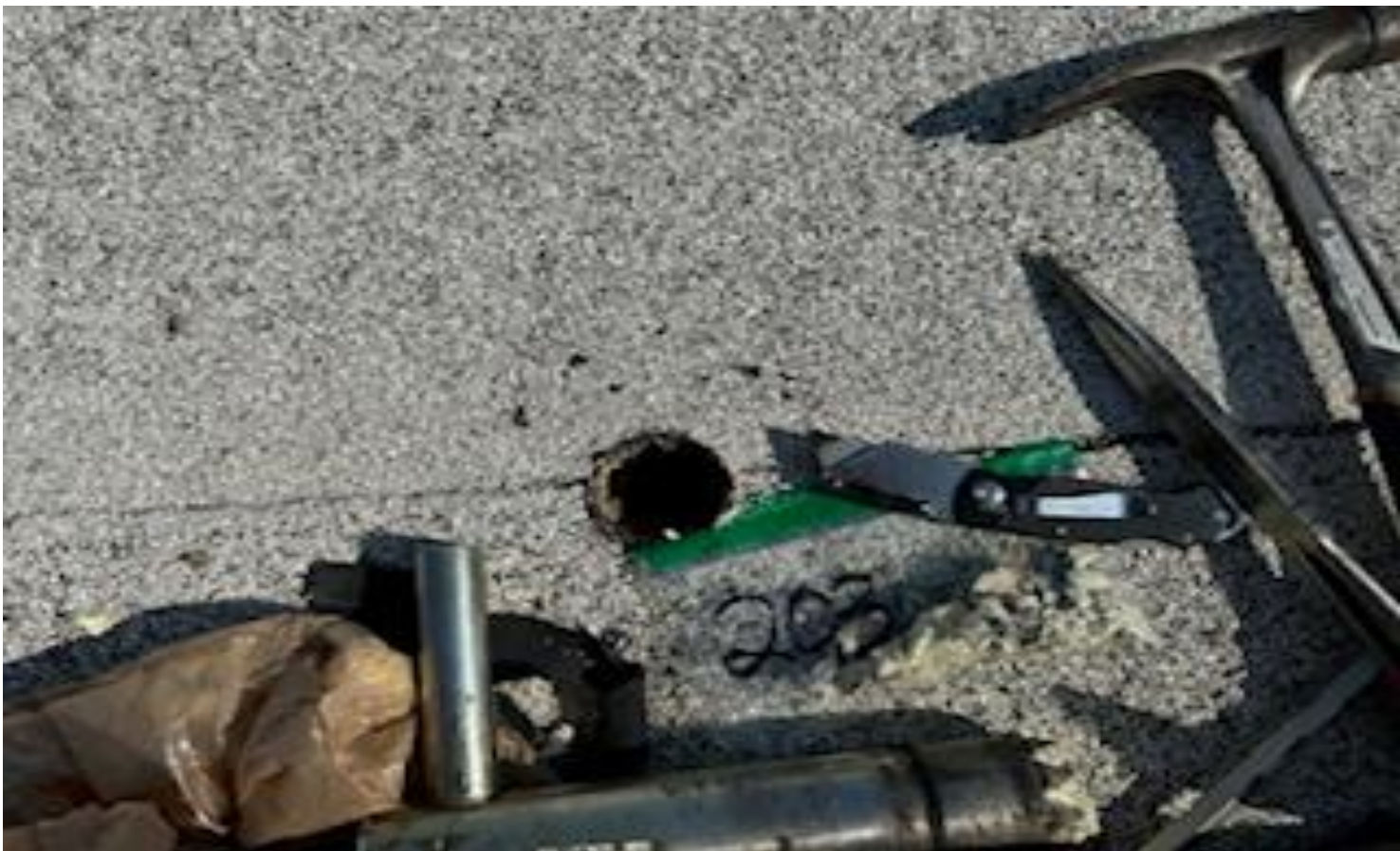
80. VIEW OF REPRESENTATIVE (TYPICAL) SAMPLE OF NON-ACM ROOF CORE PROFILE SAMPLE LOCATED THROUGHOUT TOP ROOFS OF THE BUILDINGS AT THOMAS C. MARSH PREPARATORY ACADEMY
