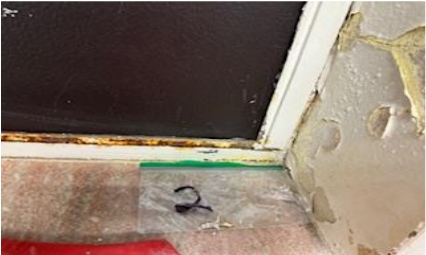
2. VIEW OF REPRESENTATIVE (TYPICAL) SAMPLE OF ACM CAULKING LOCATED ON INTERIOR WINDOW FRAMES THROUGHOUT THE BUILDINGS AT THOMAS C. MARSH PREPARATORY ACADEMY
