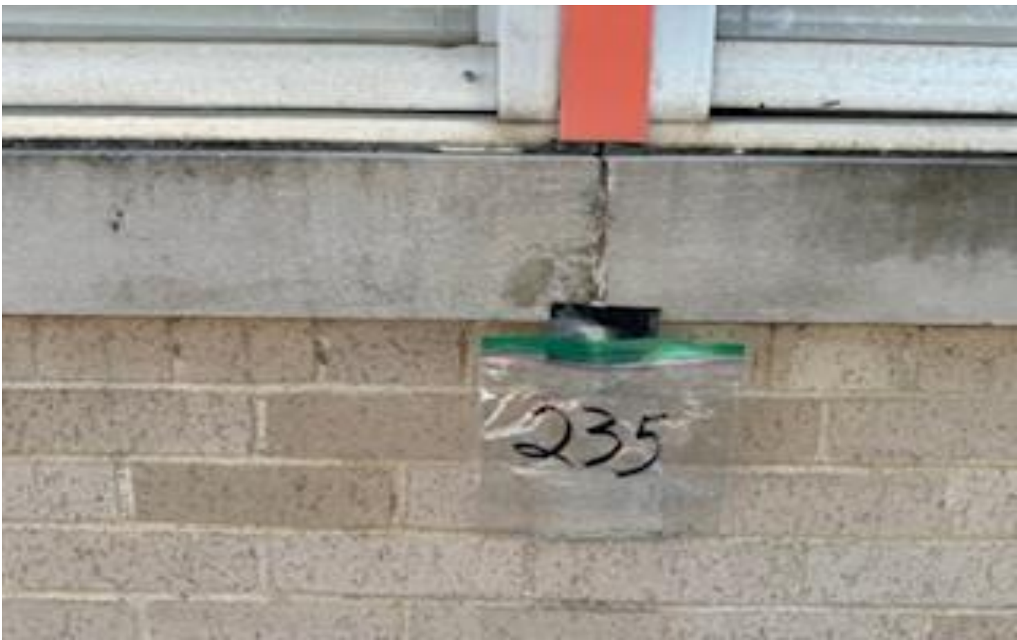
87. VIEW OF REPRESENTATIVE (TYPICAL) SAMPLE OF NON-ACM EXTERIOR CONCRETE CAULKING LOCATED AT EXTERIOR BUILDING PENETRATIONS THROUGHOUT THE BUILDINGS AT THOMAS C. MARSH PREPARATORY ACADEMY
