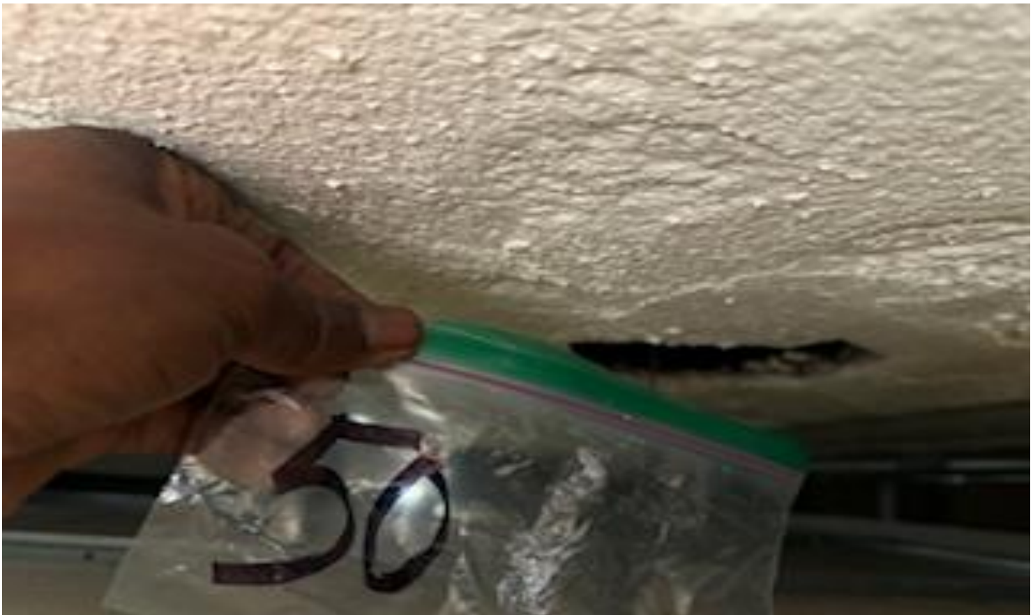
34. VIEW OF REPRESENTATIVE (TYPICAL) SAMPLE OF NON-ACM TROWELLED-ON TEXTURE ON CEILING PLASTER LATH LOCATED ON VARIOUS CEILING SURFACES IN BUILDINGS AT THOMAS C. MARSH PREPARATORY ACADEMY
