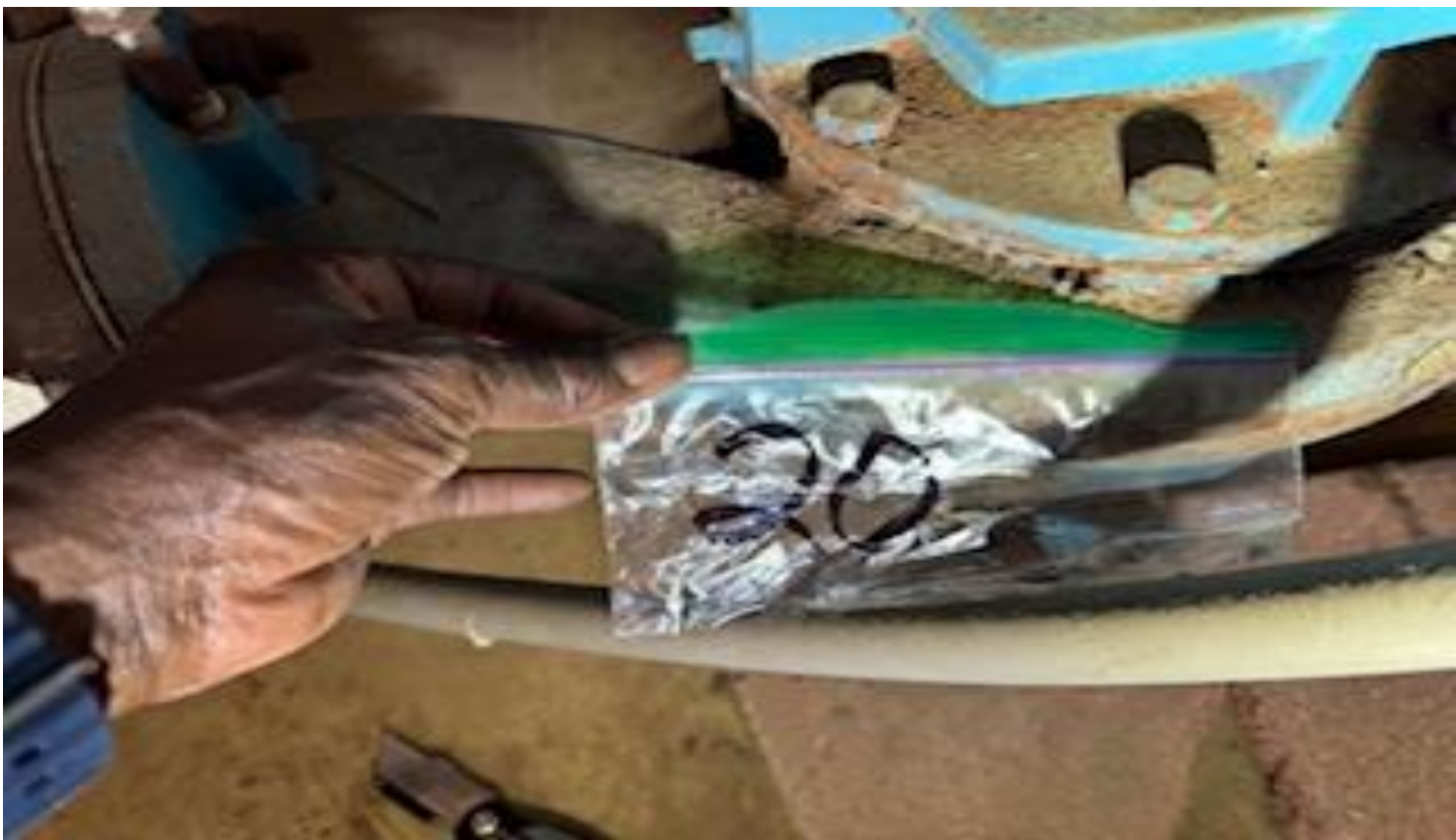
15. VIEW OF MORE REPRESENTATIVE (TYPICAL) SAMPLE OF NON-ACM GASKET INSULATION LOCATED IN THE BASEMENT BOILER/SPRINKLER ROOM IN A BUILDING AT THOMAS C. MARSH PREPARATORY ACADEMY
