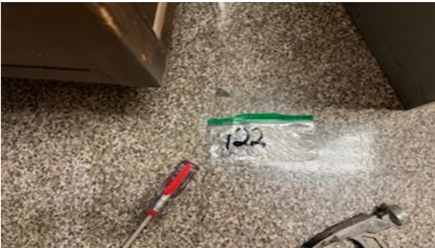
57. VIEW OF MORE REPRESENTATIVE (TYPICAL) SAMPLE OF ACM DARK BROWN 9" X 9" FLOOR TILES AND BLACK MASTIC LOCATED THROUGHOUT INTERIOR 2 ND FLOOR SURFACES IN BUILDINGS AT THOMAS C. MARSH PREPARATORY ACADEMY
