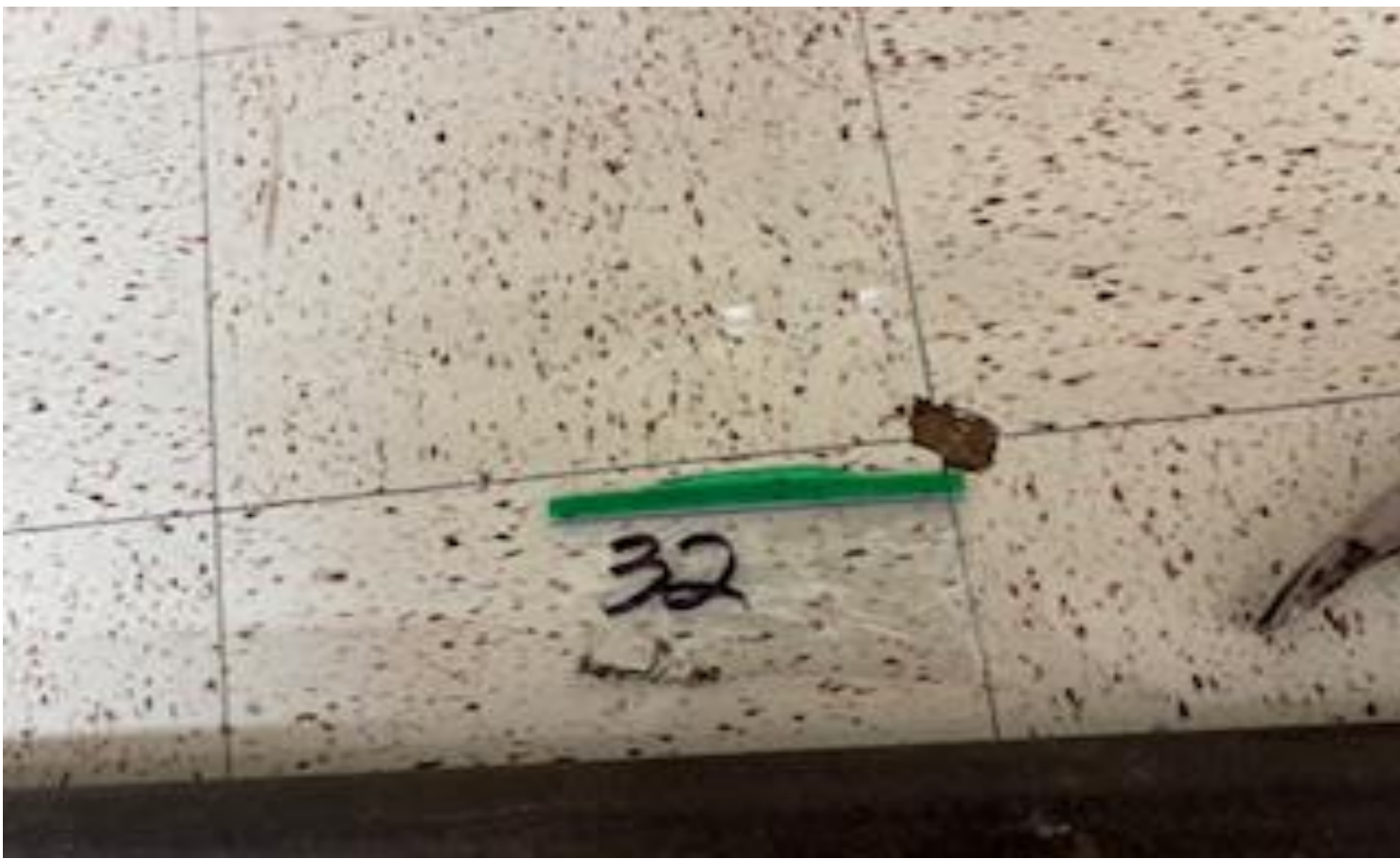
23. VIEW OF MORE REPRESENTATIVE (TYPICAL) SAMPLE OF NON-ACM 12" X12" FLOOR TILES AND MASTIC LOCATED THROUGHOUT INTERIOR FLOOR SPACES IN BUILDINGS AT THOMAS C. MARSH PREPARATORY ACADEMY
