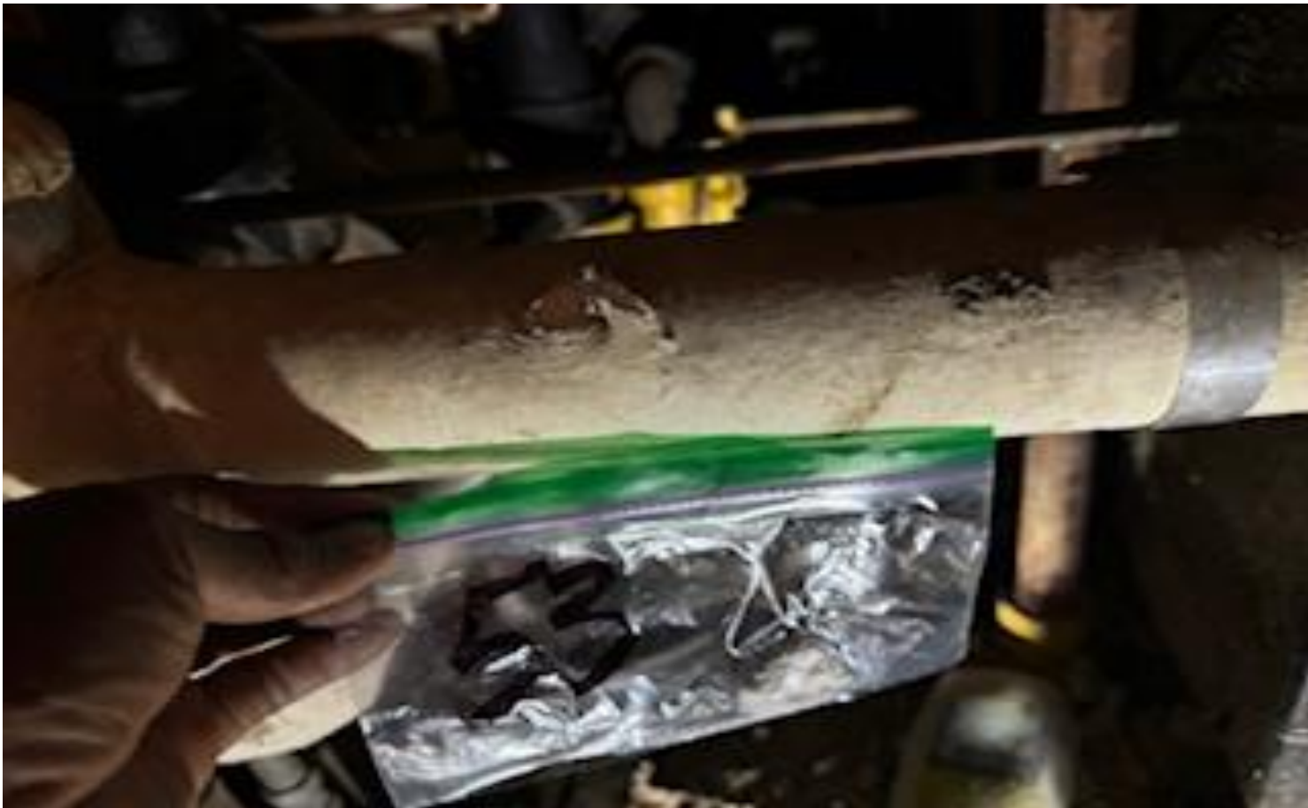
36. VIEW OF MORE REPRESENTATIVE (TYPICAL) SAMPLE OF ACM THERMAL SYSTEMS INSULATION (TSI) ON PIPE-RUNS LOCATED IN SOME AREAS IN BUILDINGS AT THOMAS C. MARSH PREPARATORY ACADEMY
