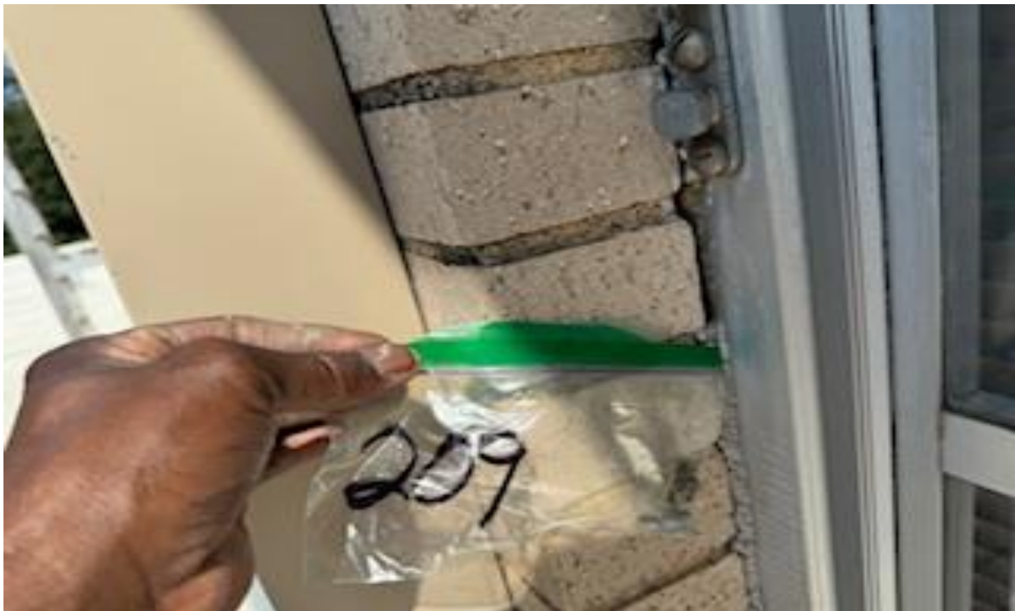
82. VIEW OF REPRESENTATIVE (TYPICAL) SAMPLE OF ACM EXTERIOR WINDOW CAULKING LOCATED THROUGHOUT THE TOP ROOFS OF BUILDINGS AT THOMAS C. MARSH PREPARATORY ACADEMY
