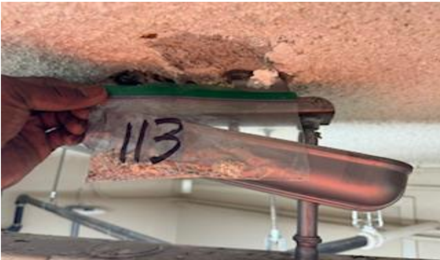
54 VIEW OF REPRESENTATIVE (TYPICAL) SAMPLE OF ACM SPRAY-APPLIED CEILING (SAC) TEXTURE LOCATED ON INTERIOR CEILING SURFACES THROUGHOUT THE BUILDINGS AT THOMAS C. MARSH PREPARATORY ACADEMY
