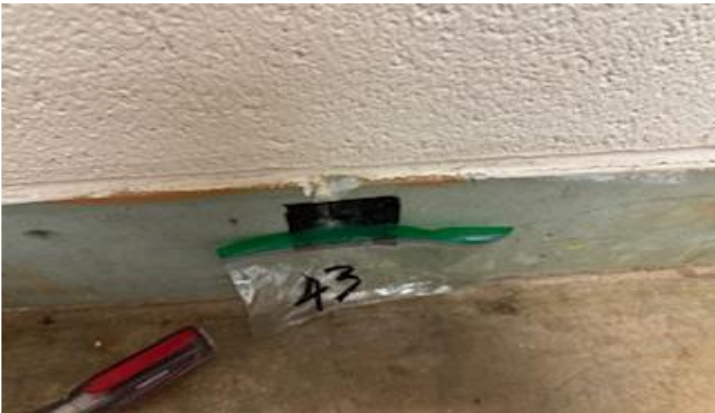
31. VIEW OF MORE REPRESENTATIVE (TYPICAL) SAMPLE OF NON-ACM GREENISH COVE-BASE CERAMIC TILES AND GROUT LOCATED THROUGHOUT THE BUILDINGS AT THOMAS C. MARSH PREPARATORY ACADEMY
