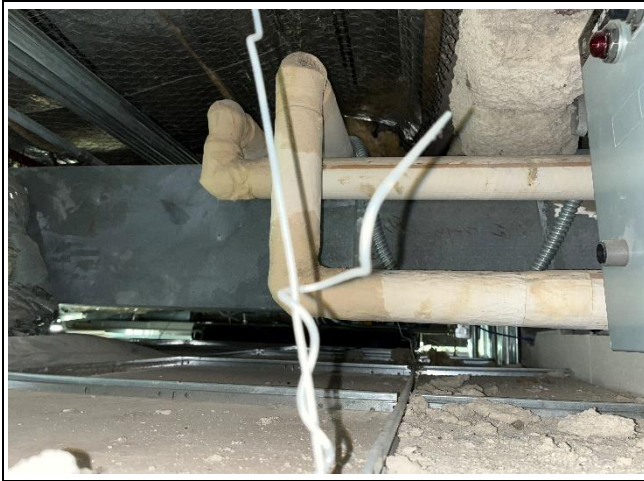
Photo 03: ACM Heating water pipe insulation with cream mastic
