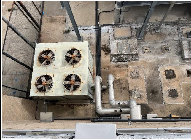
Photo 05: Air-cooled chiller and pipe insulation – nonACM
