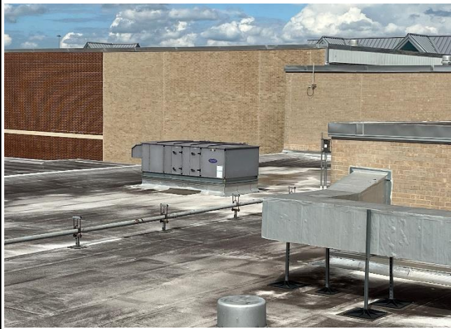
Photo 05: RTU with chilled / heating water pipe insulation – nonACM.
