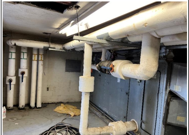
Photo 06: Penthouse mechanical room – nonACM pipe insulation and duct sealant.
