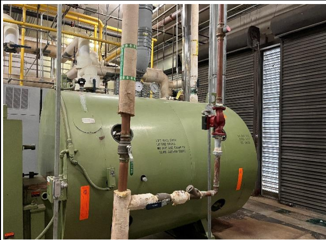
Photo 05: Domestic water boiler - nonACM
