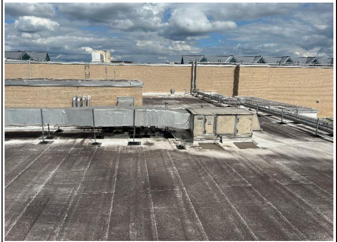
Photo 06: RTU with duct insulation and chilled / heating water pipe insulation – nonACM.
