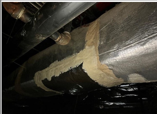
Photo 01: ACM Tan/cream mastic on duct insulation
