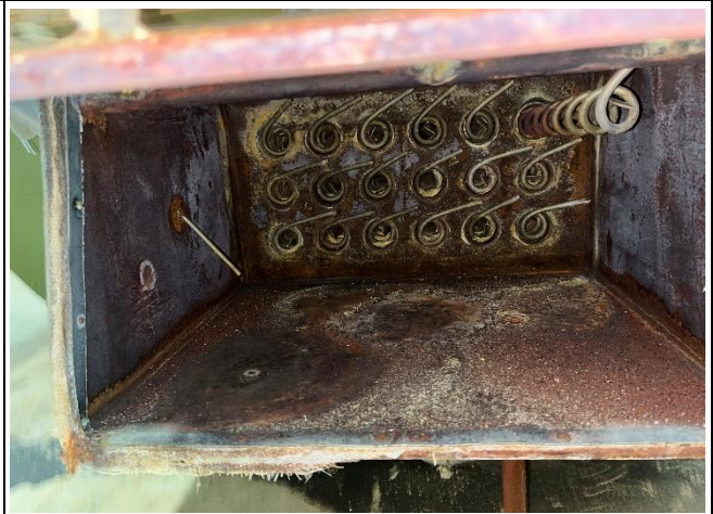
Photo 06: Domestic water boiler – nonACM
