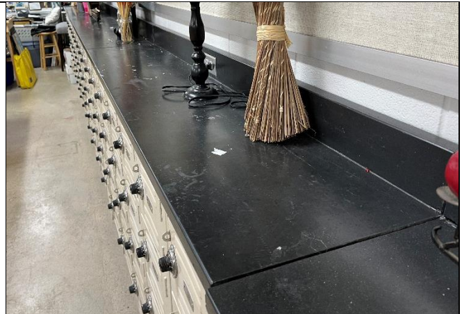
Photo 02: ACM Transite Countertop in Art Room
