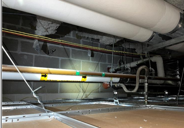
Photo 03: Domestic cold water – un-insulated.
