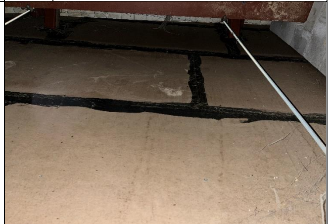
Photo 04: ACM Black mastic damp proofing on gyp-board sheathing behind brick veneer.
