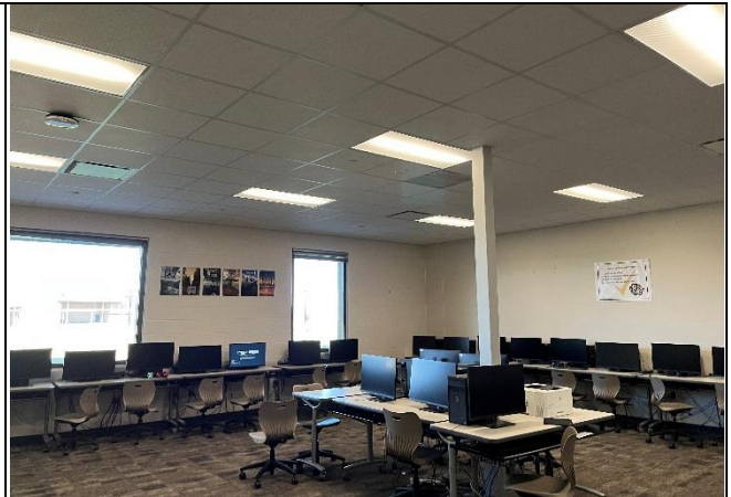
Photo 02: 2'x2' Pinhole ceiling panels, carpet pad and glue, cove base - typical - nonACM
