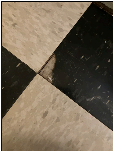
7 - Typical floor tile sample
