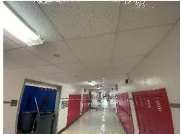
Photo #2 View of non-asbestos containing 2' x 2' ceiling tile (pins and small fissure).
