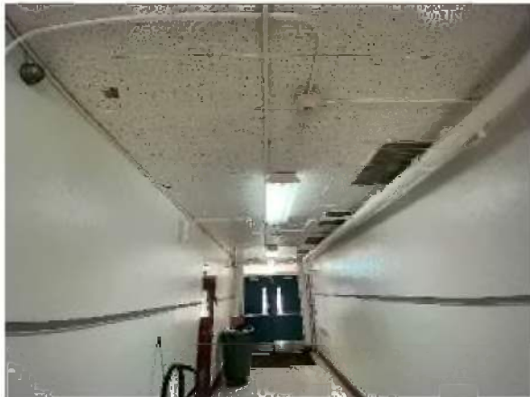
Photo #3 View of the non-asbestos containing Plaster walls and 12" x 12" ceiling tile.
